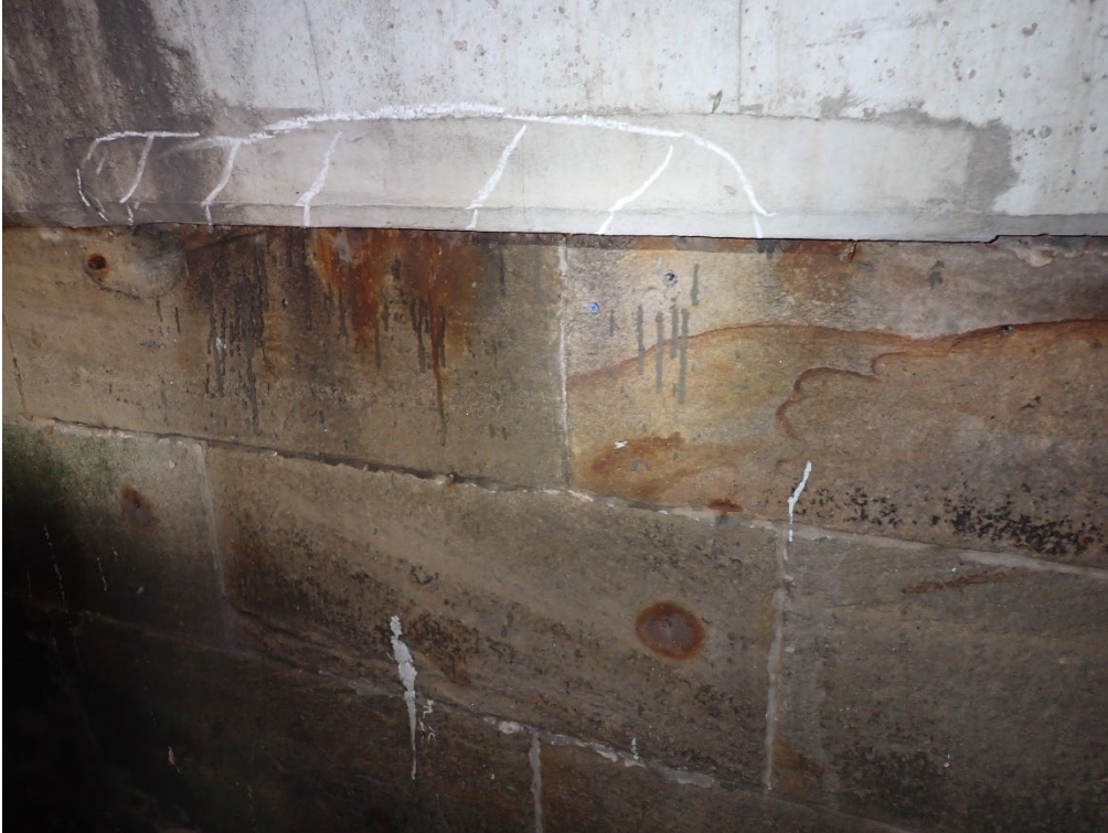
Plate 81. Typical minor mortar loss to the Centre Pier
