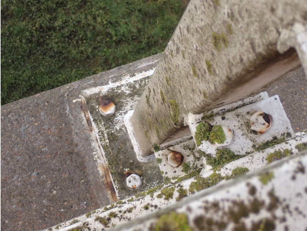
Plate 163. Typical Rust Staining to Parapet post base plates
