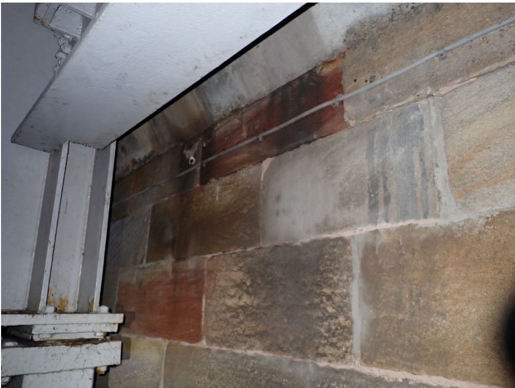
Plate 36. Water staining to the West Abutment back wall
