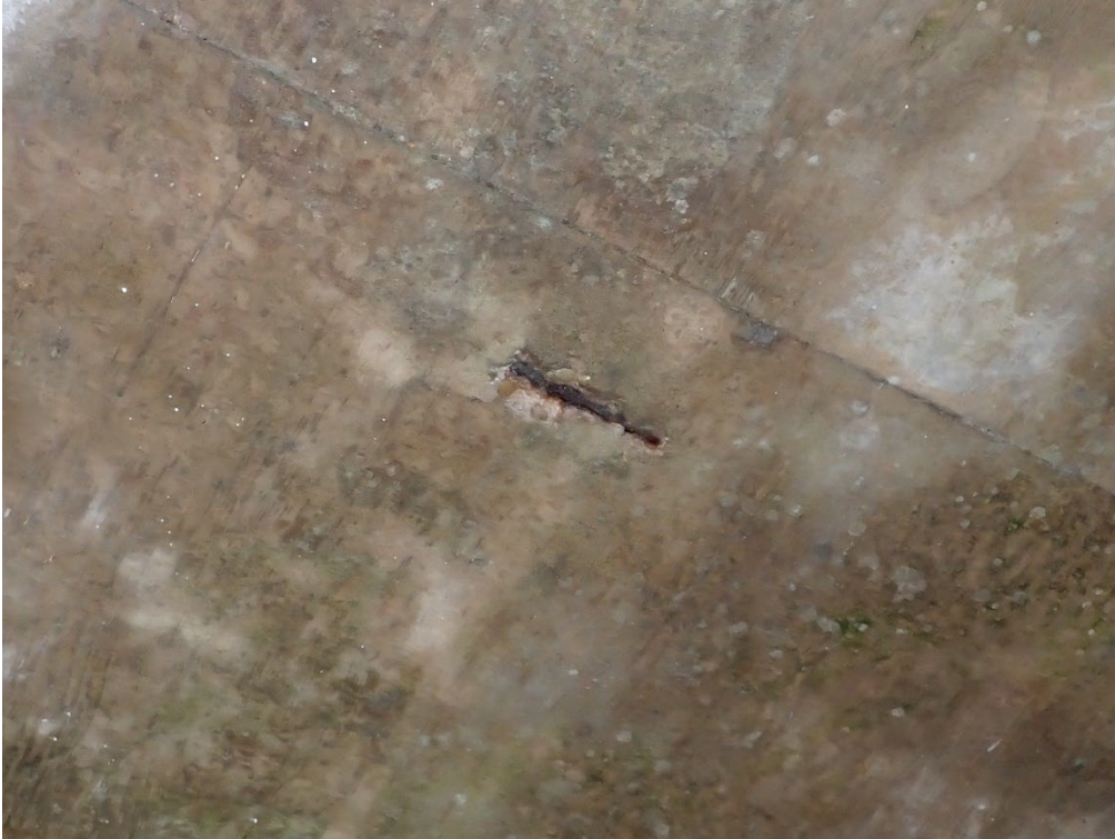
Plate 117. Exposed reinforcement in East Span
