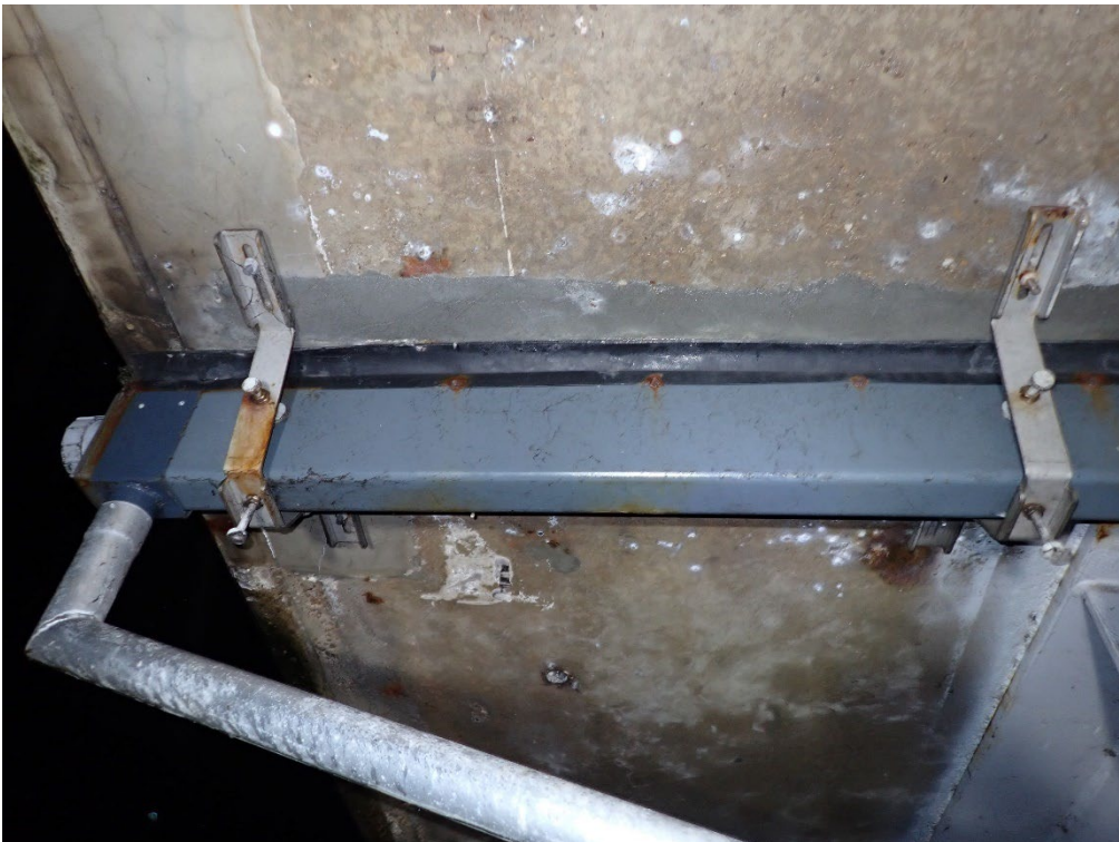
Plate 128. Minor corrosion to fixings on the East Joint
