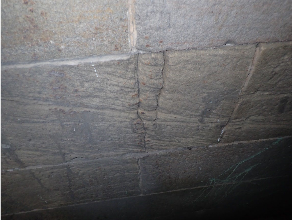
Plate 79. Crack Through Stone in the West Pier
