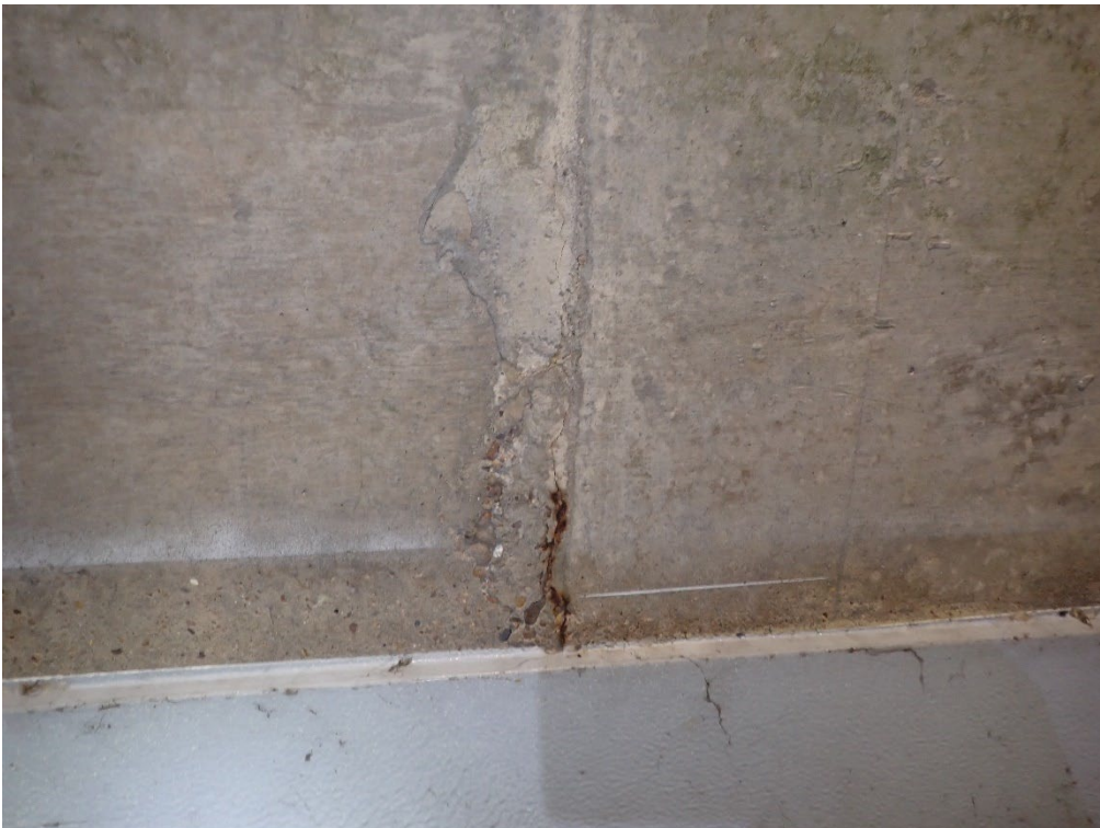
Plate 118. Corroded ferrous debris & crack, North edge beam on West Span
