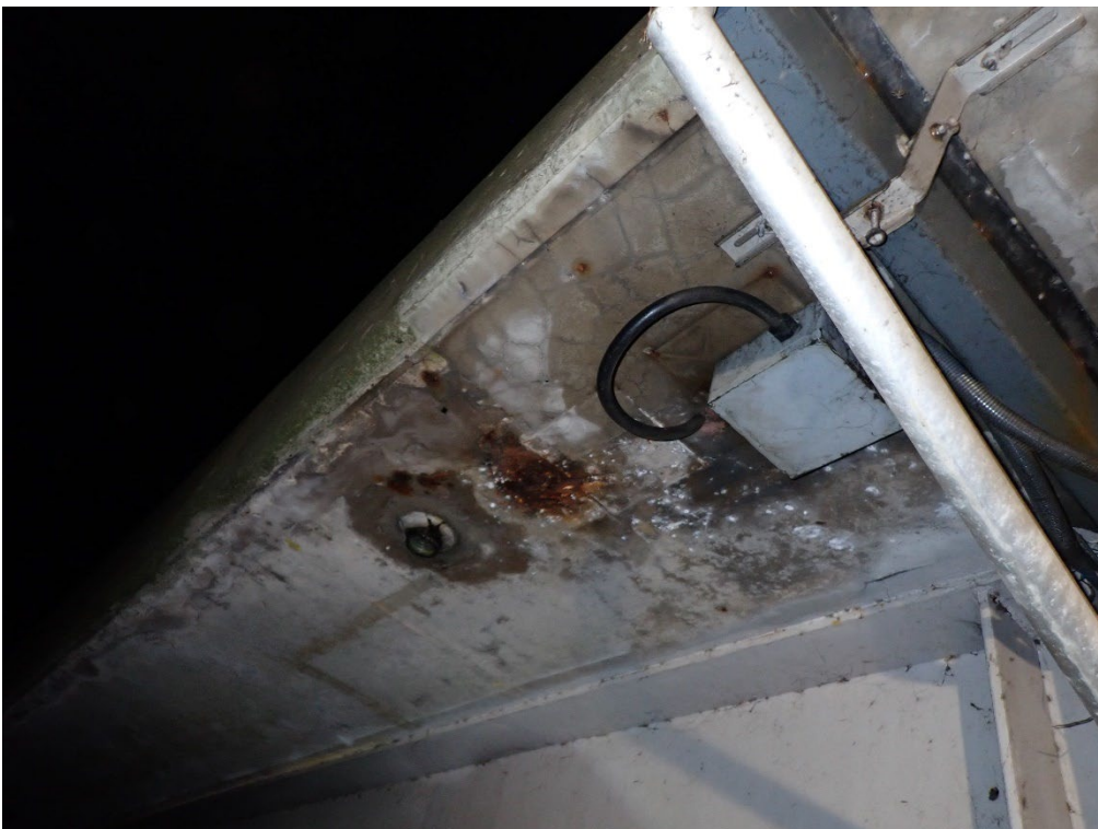
Plate 106. Minor spalled concrete and cracked repair to the North edge beam adjacent the West Joint
