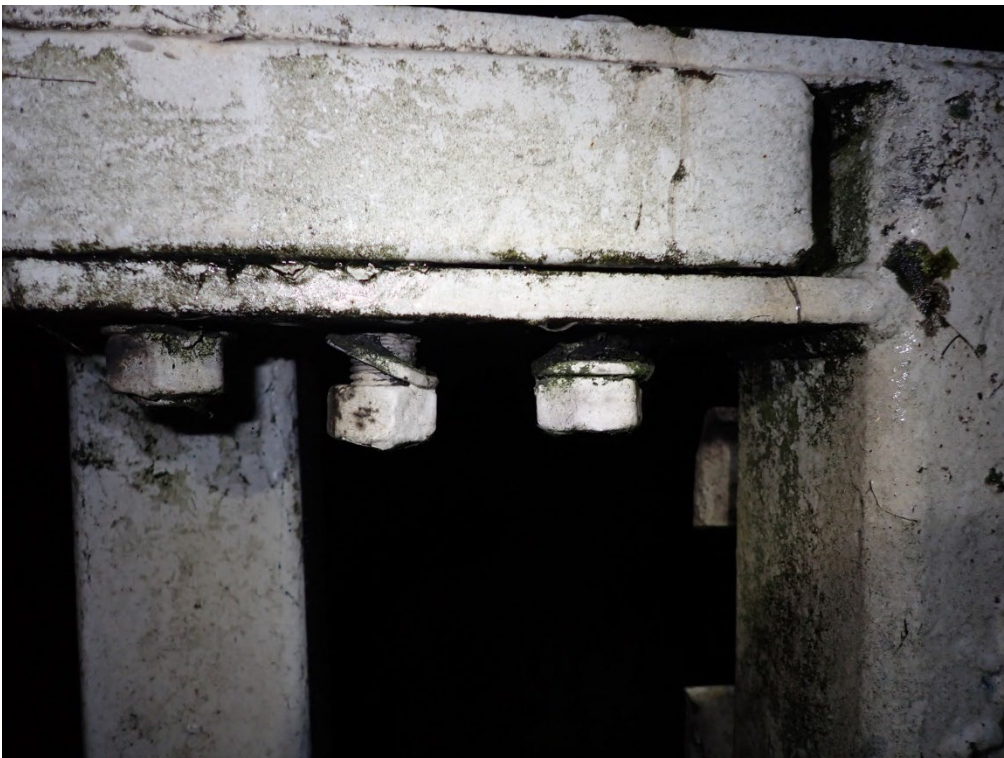
Plate 170. Loose nuts on the connection at the North-East corner
