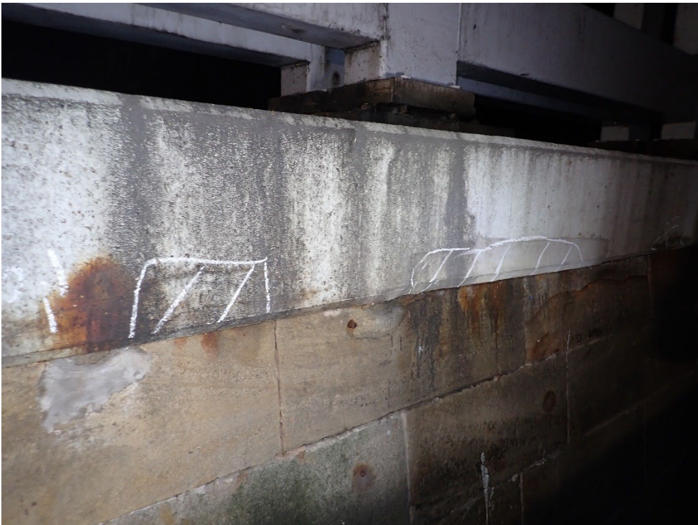
Plate 66. Two areas of delamination, Centre Pier measured up to 920 x 120mm.
