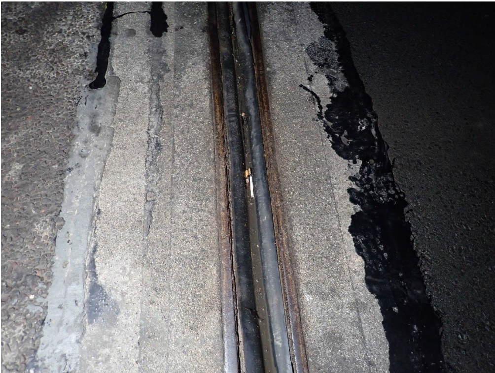
Plate 156. Debris within the Centre Pier joint seal
