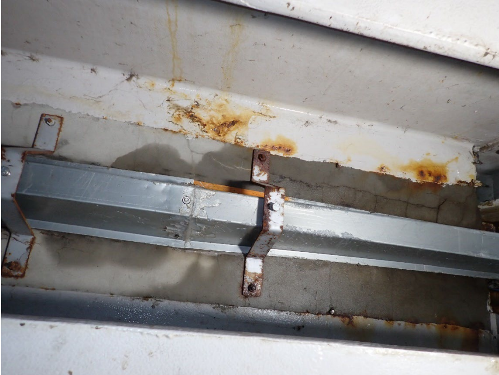
Plate 129. Corrosion to fixings on the Centre Pier joint drainage
