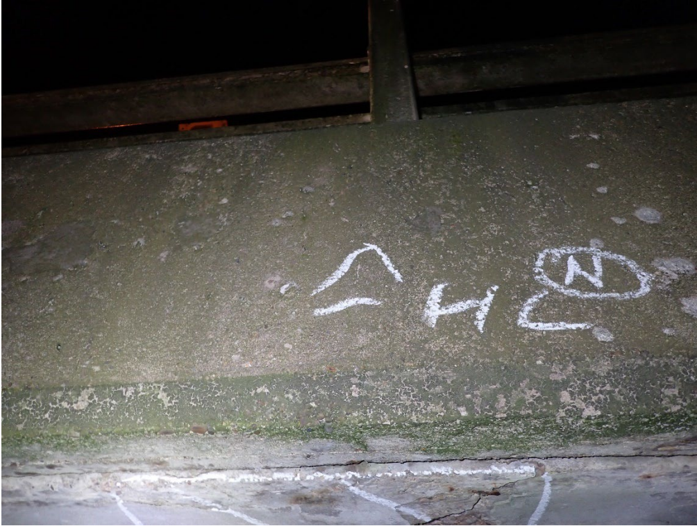
Plate 121. Hairline cracking North edge beam, West Span
