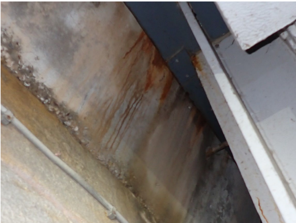
Plate 42. Rust staining emanating from the drainage deflector on the West Abutment
