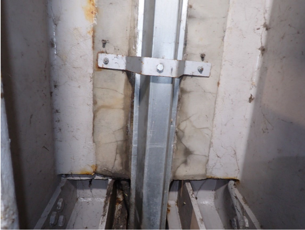
Plate 139. Cracking to a repair beneath the West Joint
