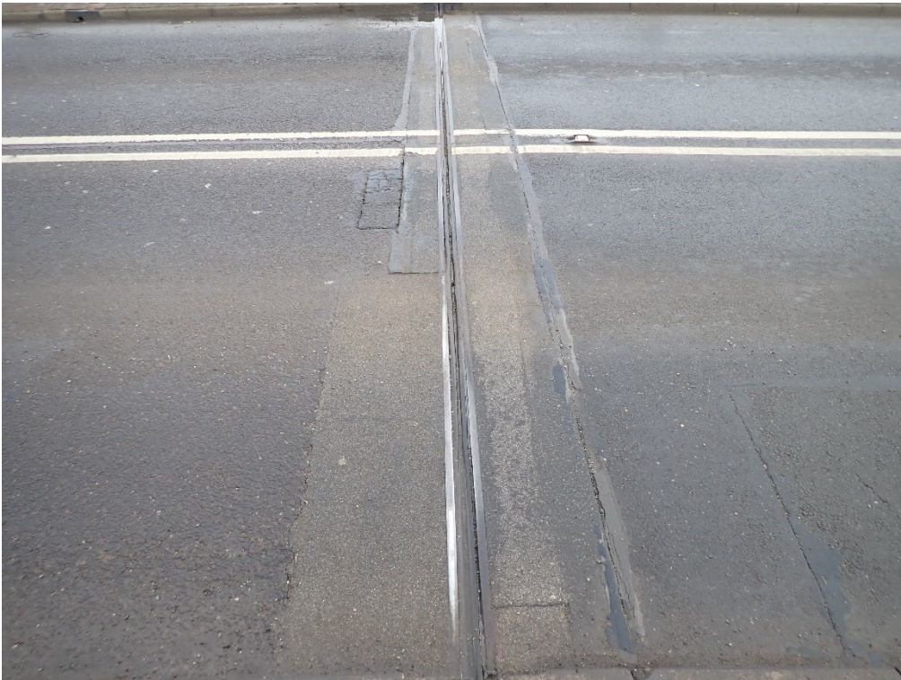
Plate 144. Failed repair and cracking adjacent the East Abutment joint
