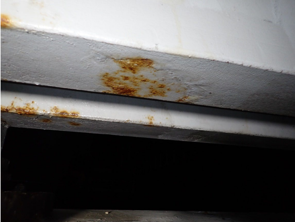
Plate 91. Minor corrosion to the centre Pier cross beam
