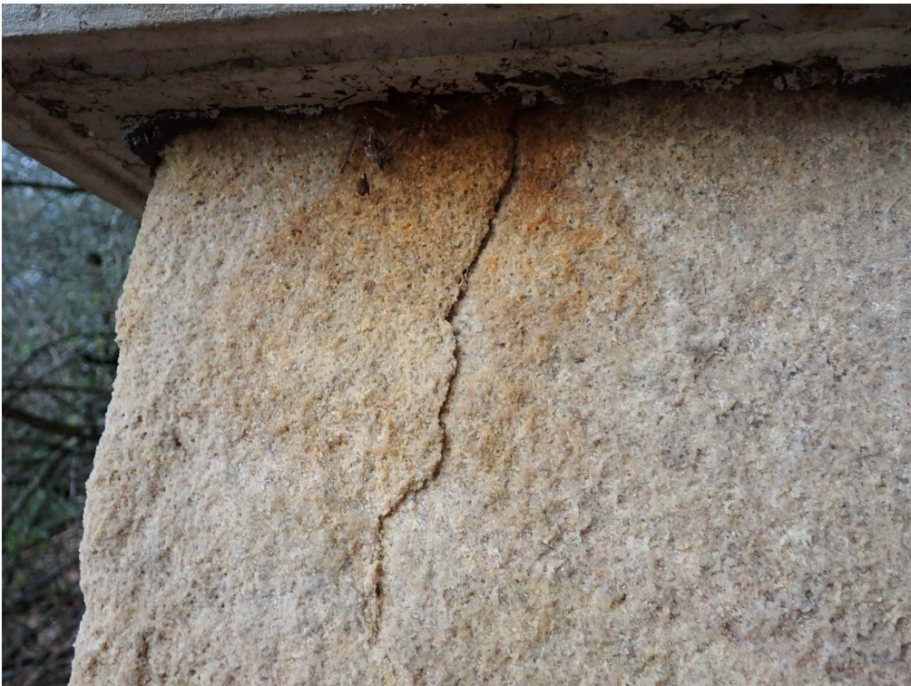
Plate 50. Cracking through stones in the West Abutment lower wall
