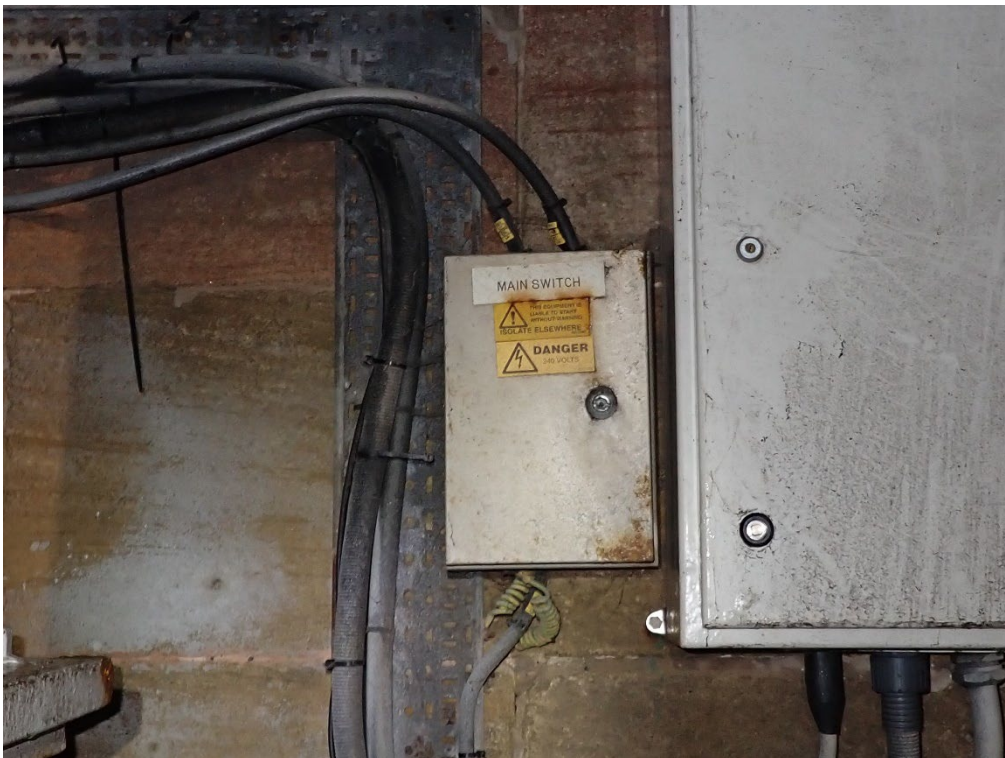
Plate 58. Minor corrosion to the cathodic protection cabinet on the East Abutment back wall
