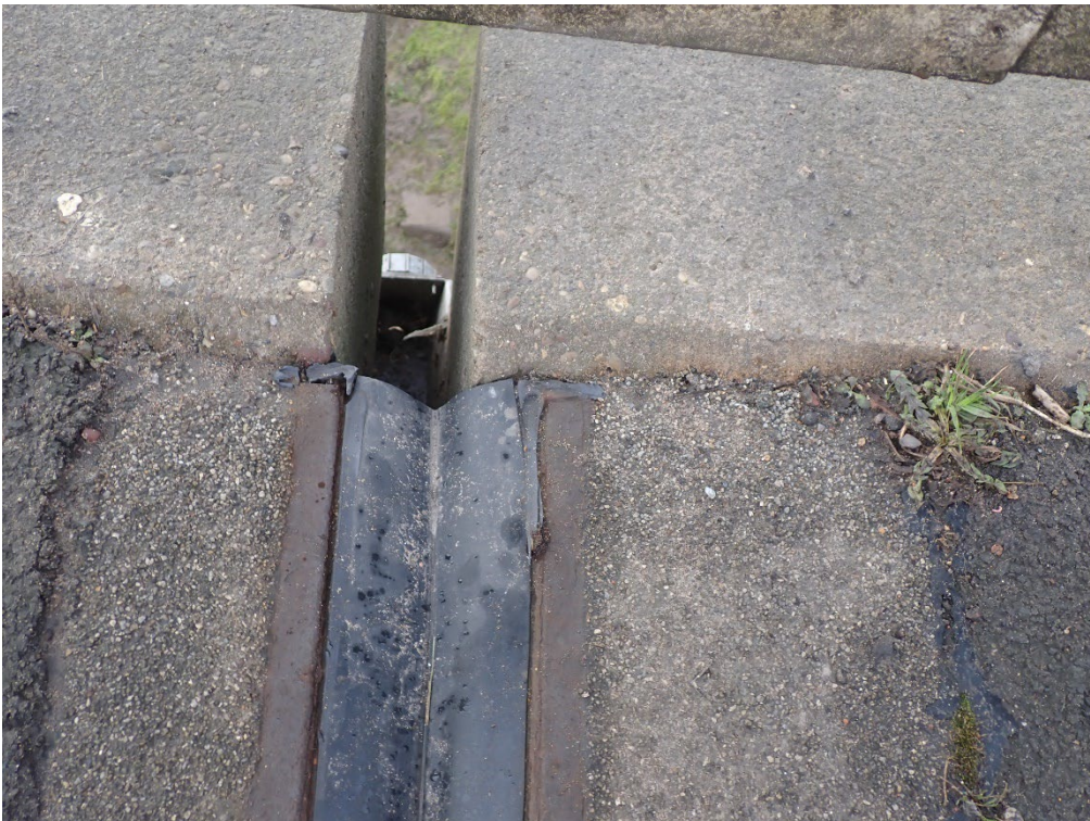
Plate 124. No sealant in joint above the Centre Pier
