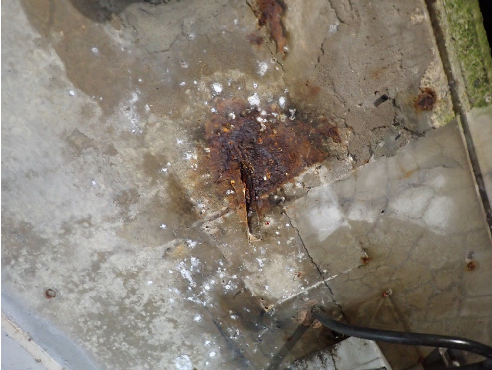
Plate 107. Minor spall and cracked repair to the North edge beam on the West inner span
