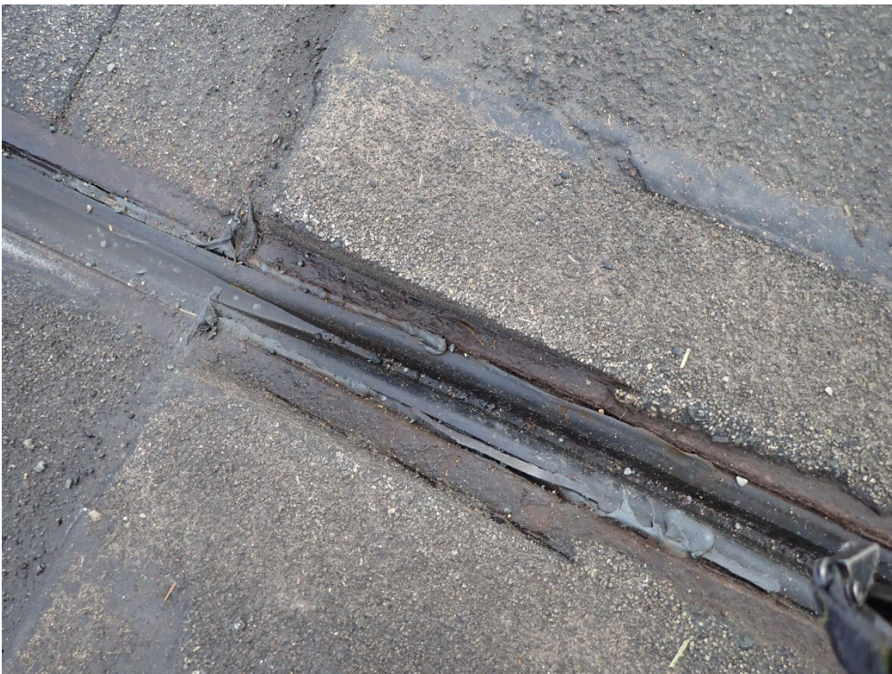
Plate 152. Corrosion with lamination to the East Joint rails
