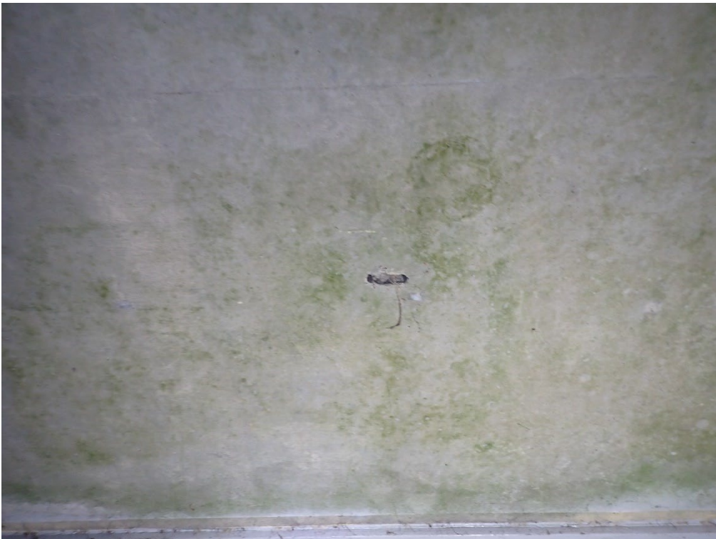
Plate 126. Void in Deck Soffit, Inner West Span
