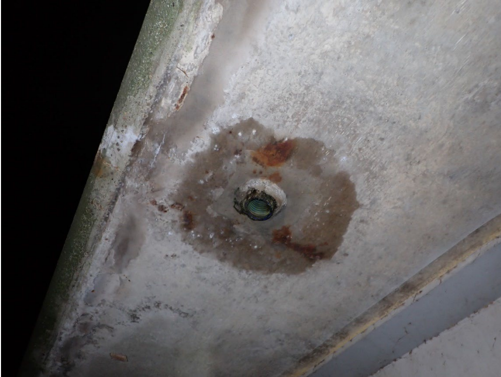
Plate 113. Rust staining adjacent to deck drainage outlet
