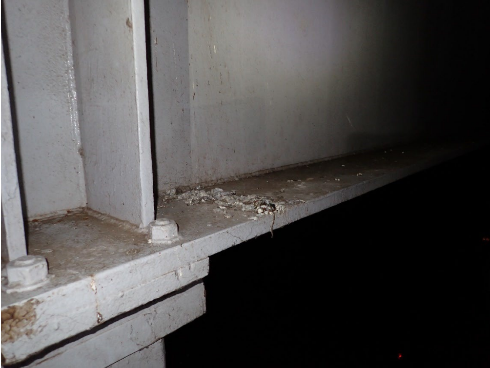
Plate 103. Bird dropping to the South edge beam adjacent the East Pier
