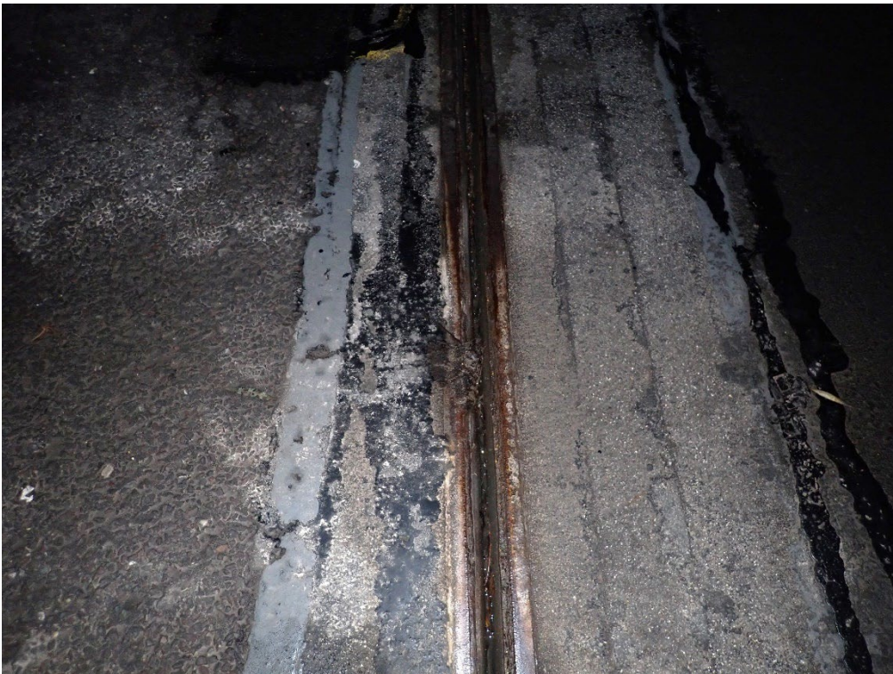
Plate 148. Non-Continuous & untidy Joint in the nosing rails, West Abutment
