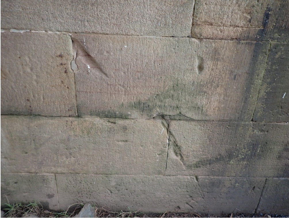
Plate 73. Impact Scraping to the West Pier
