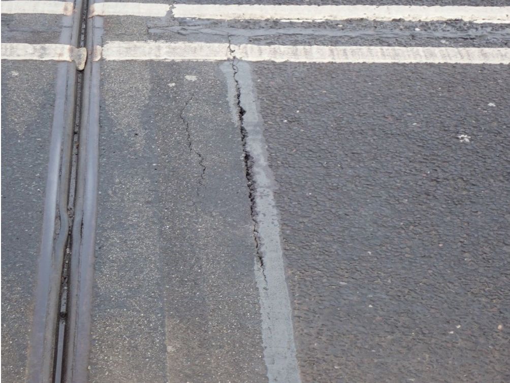
Plate 147. Cracking in the nosing material of the East Pier joint
