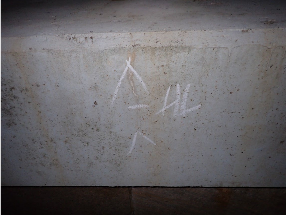
Plate 69. Cracking to the East Pier concrete cap
