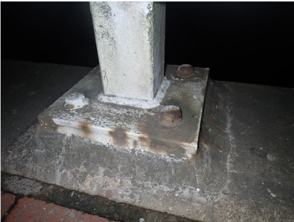
Plate 164. Typical corrosion and rust staining to North Parapet post base plate
