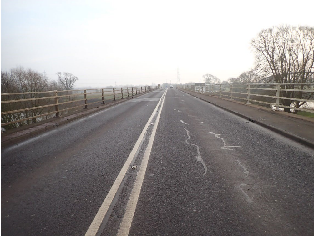
Plate 137. Typical carriageway condition, Inner West Span
