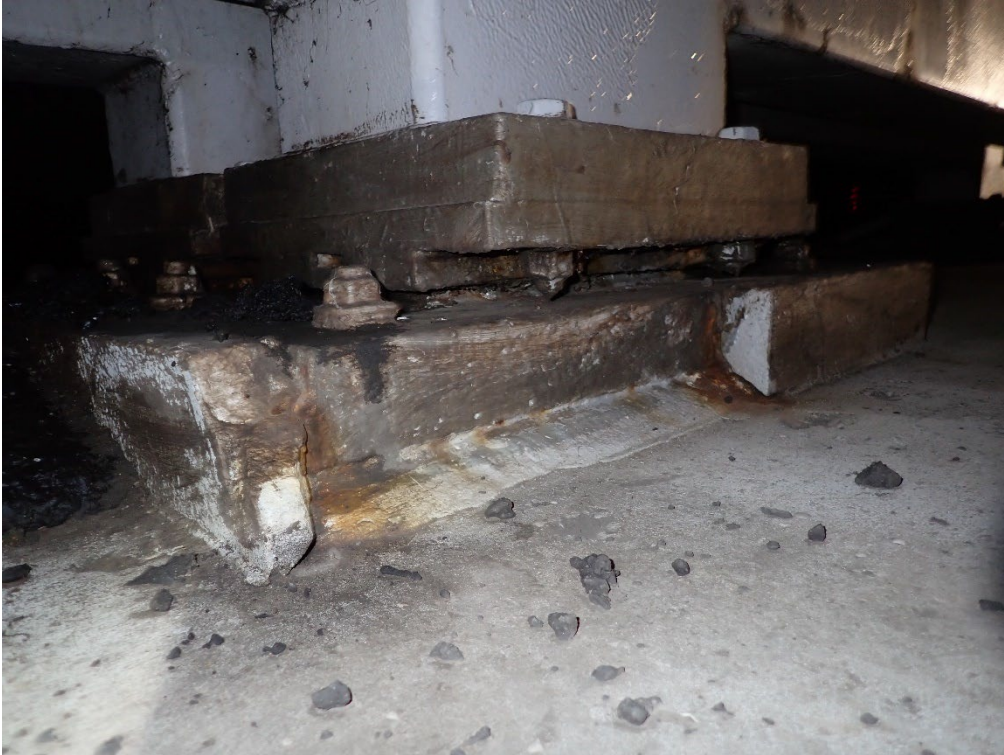
Plate 93. Spalling to the lower bearing plinth on the Centre Pier
