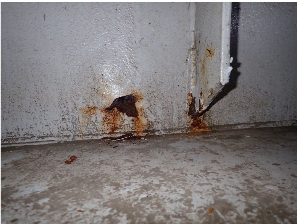
Plate 96. Flaking paint exposing underlying corrosion to South Beam, West Span
