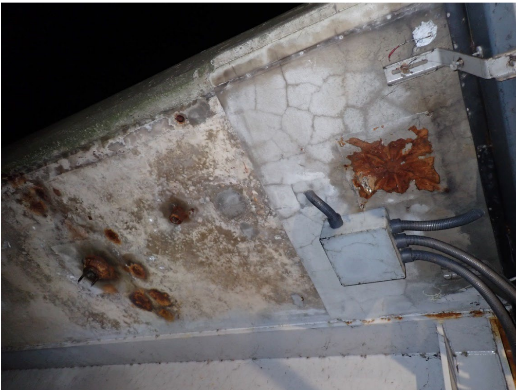
Plate 110. Minor spall and cracked repair to the North edge beam adjacent the East Joint
