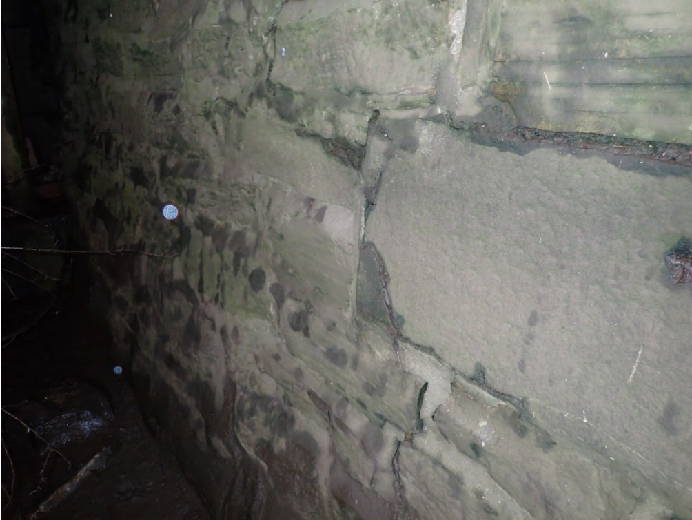
Plate 173. Vertical crack in the North Face of the South Retaining Wall
