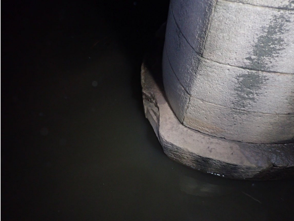
Plate 71. Spall to Downstream End of the Centre Pier
