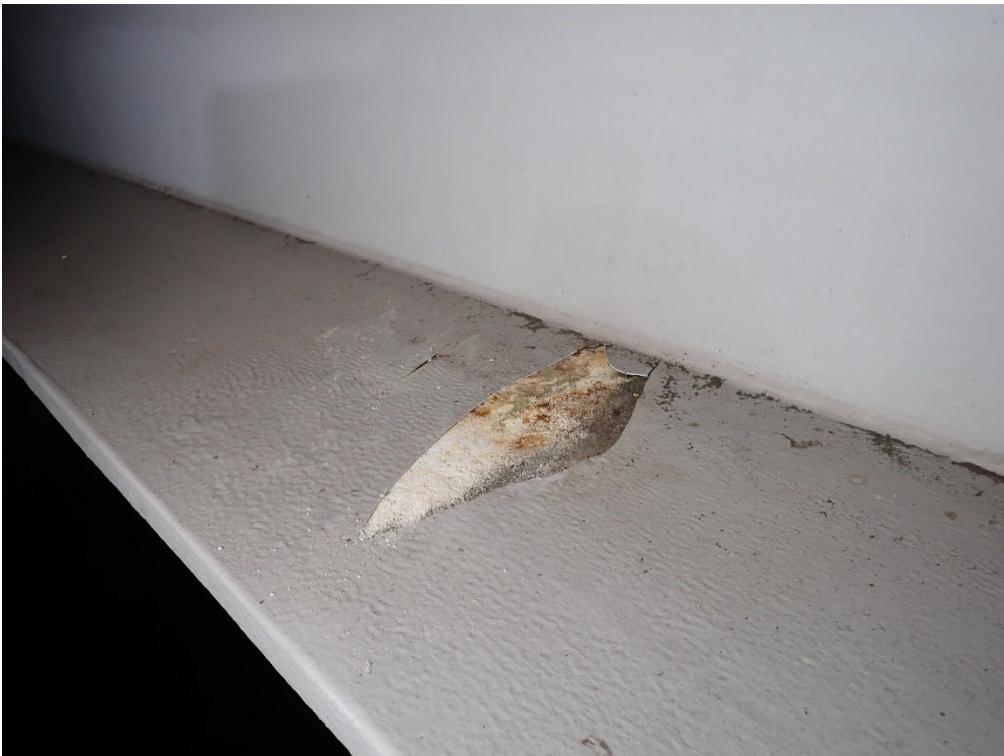
Plate 98. Flaking Paint to South Beam, Inner West Span
