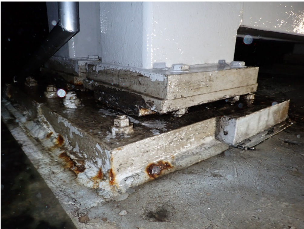
Plate 92. Spalling to the lower bearing plinth on the East Pier
