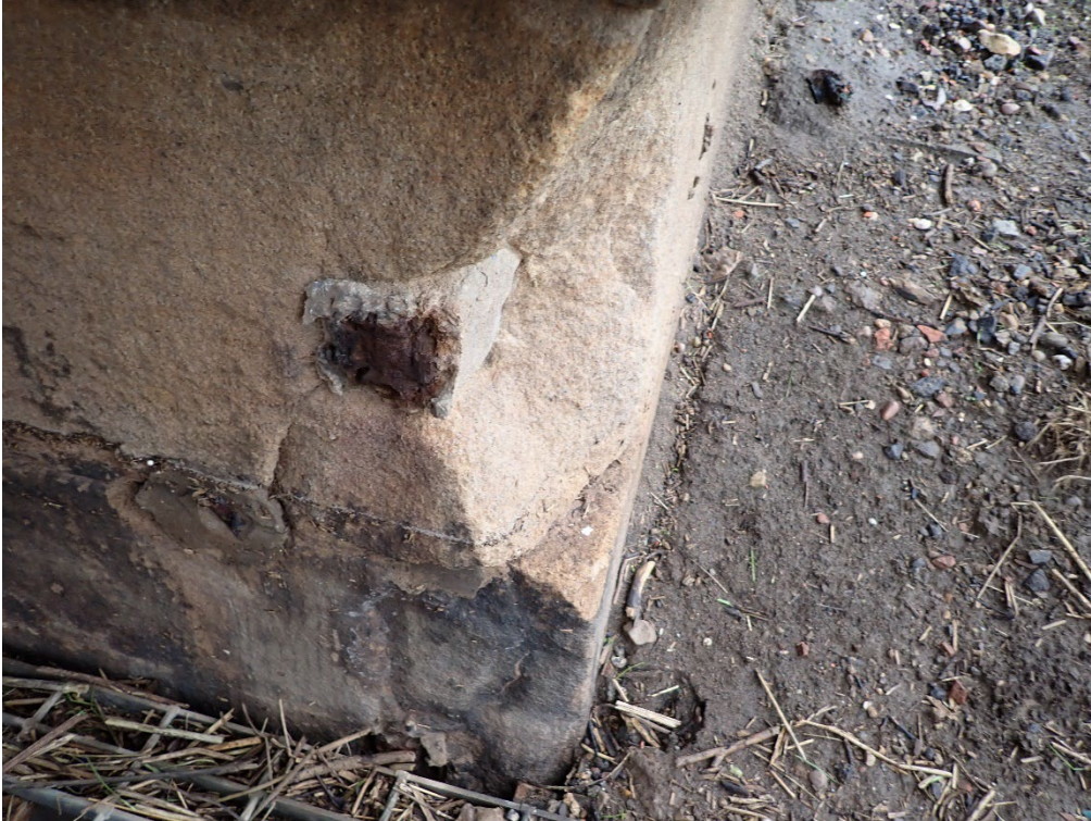
Plate 47. Spall to stone in the East Abutment adjacent to historic fixing, 300 x 10 x 40mm.
