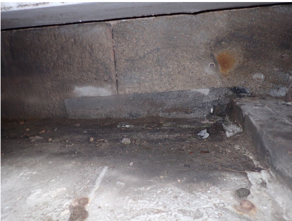
Plate 56. Damage to felt on the West Abutment
