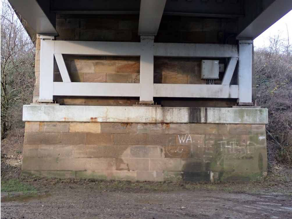
Plate 59. Painted Graffiti on the West Abutment
