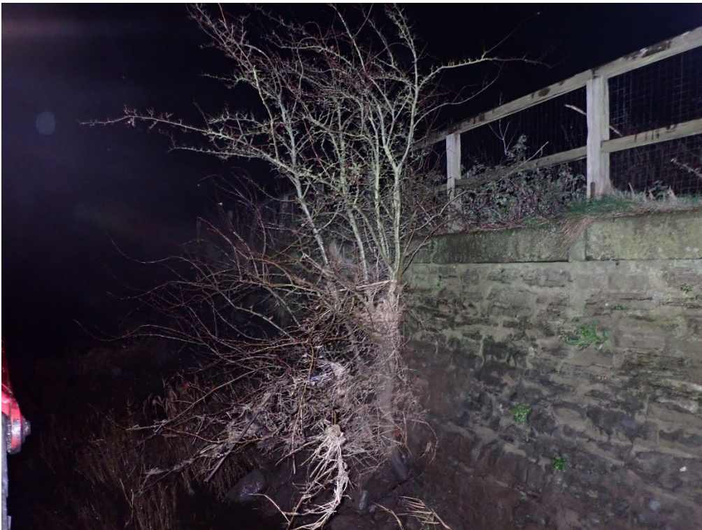
Plate 174. Tree growth at the base of the North-East Retaining Wall
