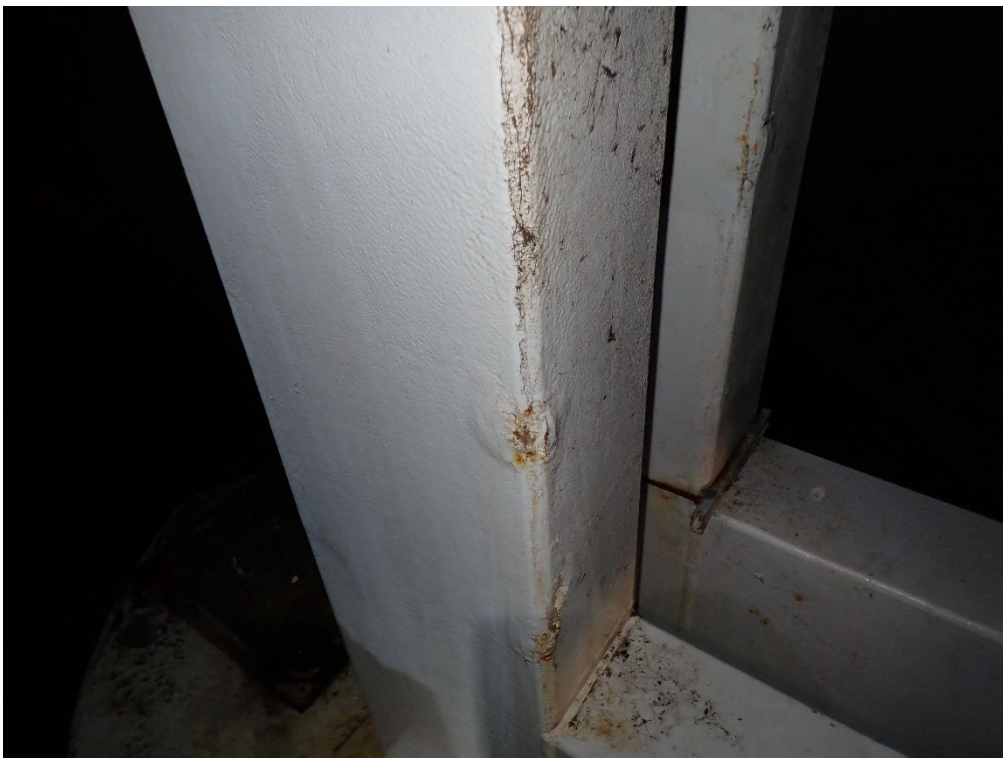
Plate 86. Paint blistering within the West Pier bearing frame
