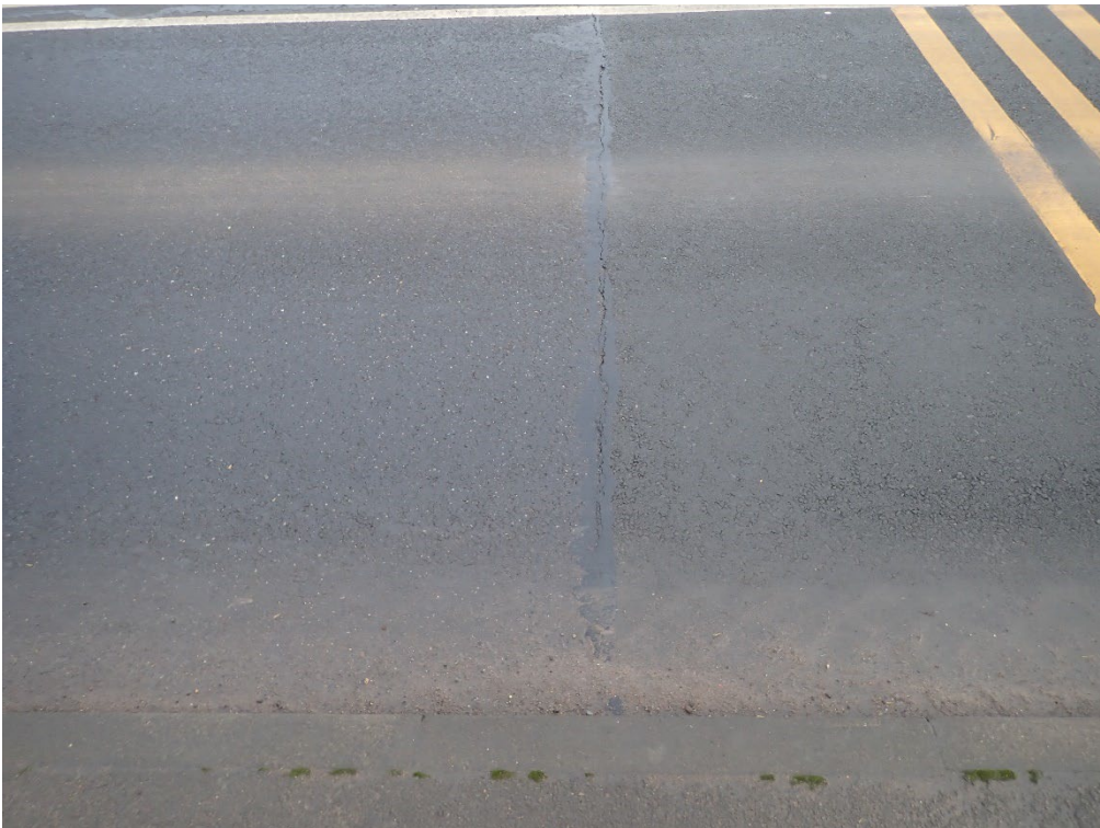
Plate 132. Transverse cracking on the East Approach
