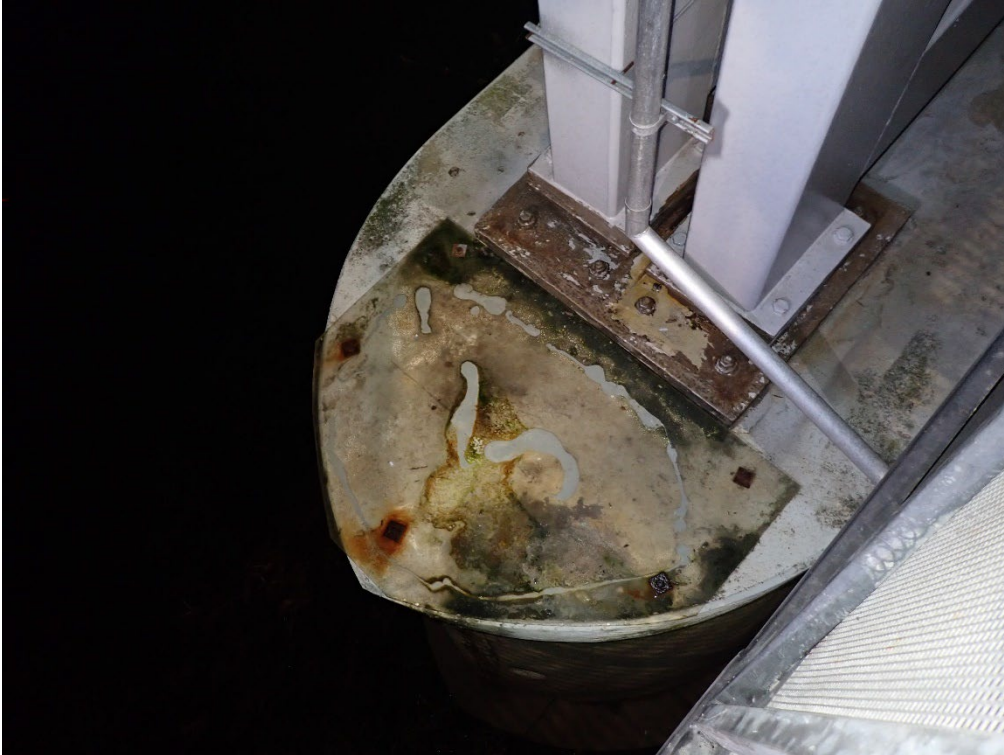
Plate 75. Water staining to upstream end of the Centre Pier
