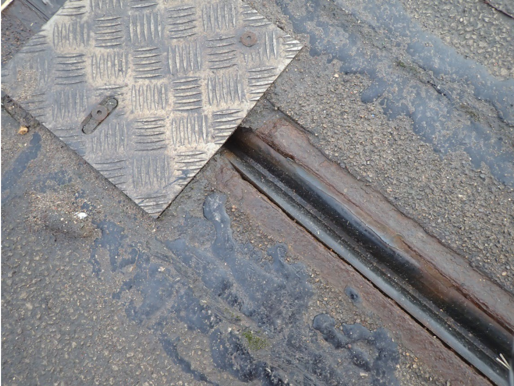
Plate 149. Corrosion and minor lamination to the West Abutment joint rails
