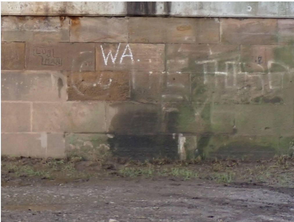
Plate 60. Historic fire damage to the West Abutment
