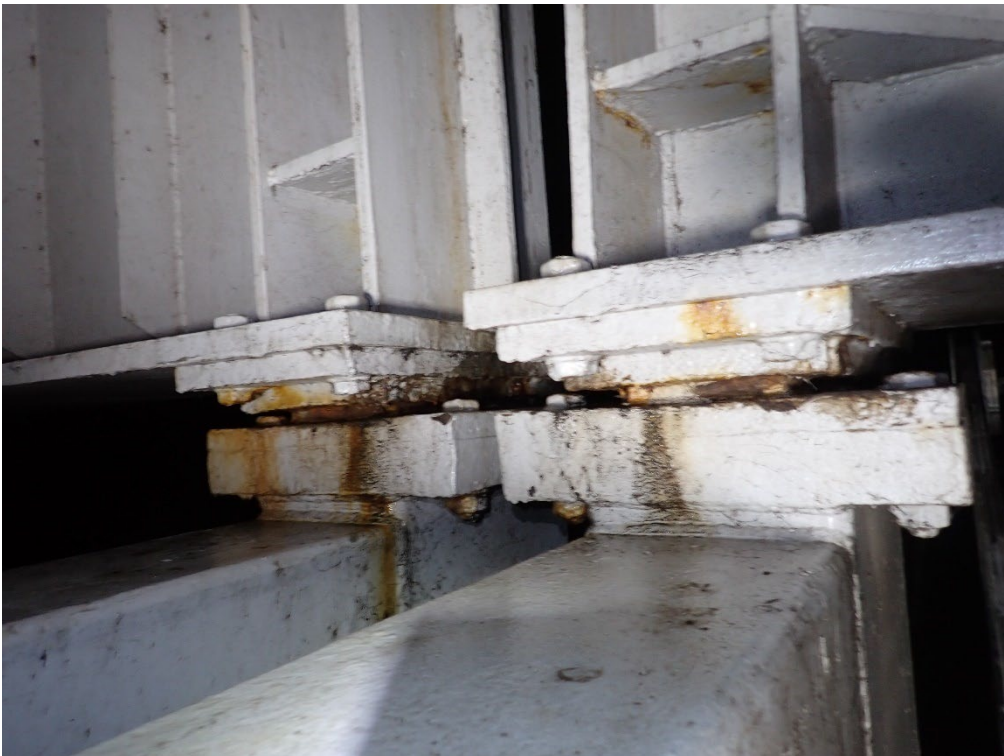
Plate 88. Spalled grout around Centre Pier Bearing
