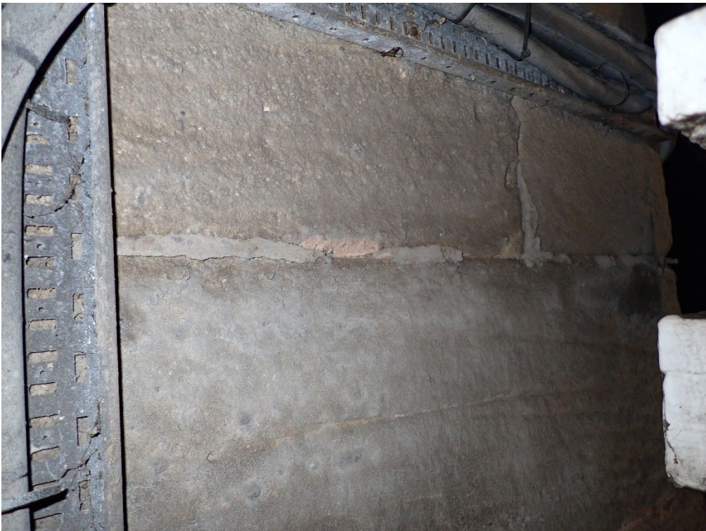
Plate 52. Typical condition of mortar on the West Abutment back all
