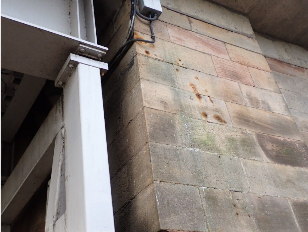
Plate 63. Corroded Historic Fixings, North-West Wing Wall
