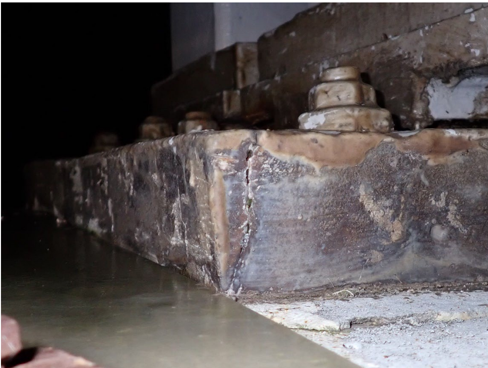
Plate 94. Cracking to the Centre Pier bearing plinth
