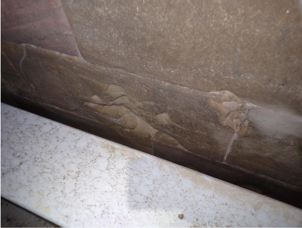
Plate 45. Shallow spall to West Abutment stone
