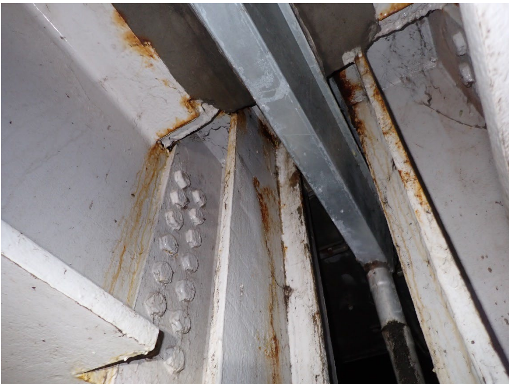
Plate 100. Corrosion staining to steelwork above the Centre Pier
