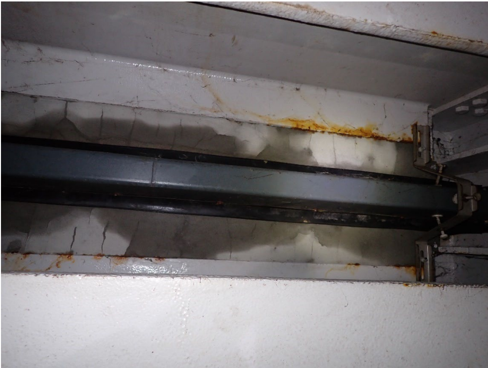
Plate 140. Water seepage and cracking to the repair beneath the Centre Pier joint
