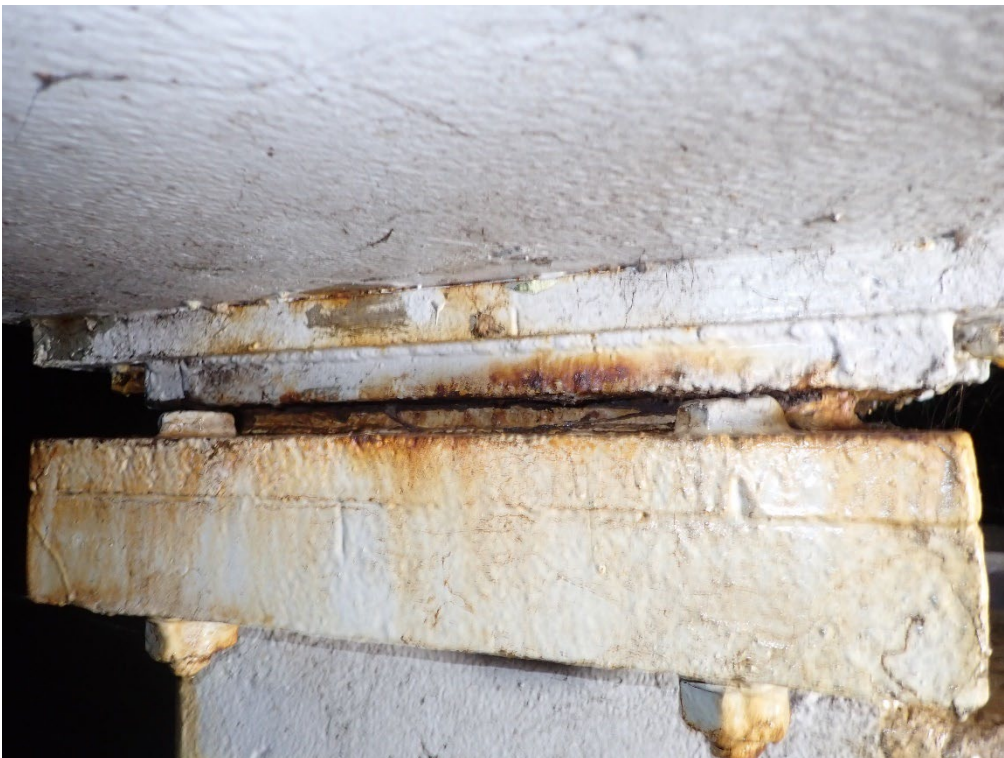
Plate 90. Paint blistering and cession to the South upper bearing on the Centre Pier
