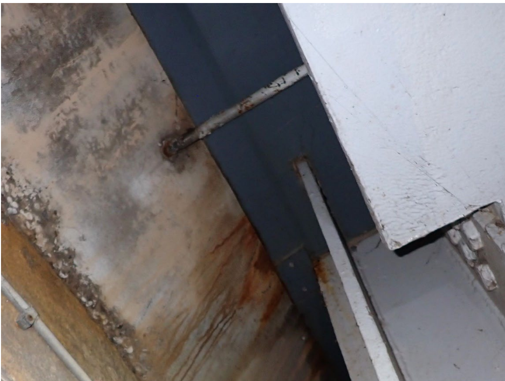
Plate 44. Minor corrosion from paint loss on the anchorage bar at West Abutment
