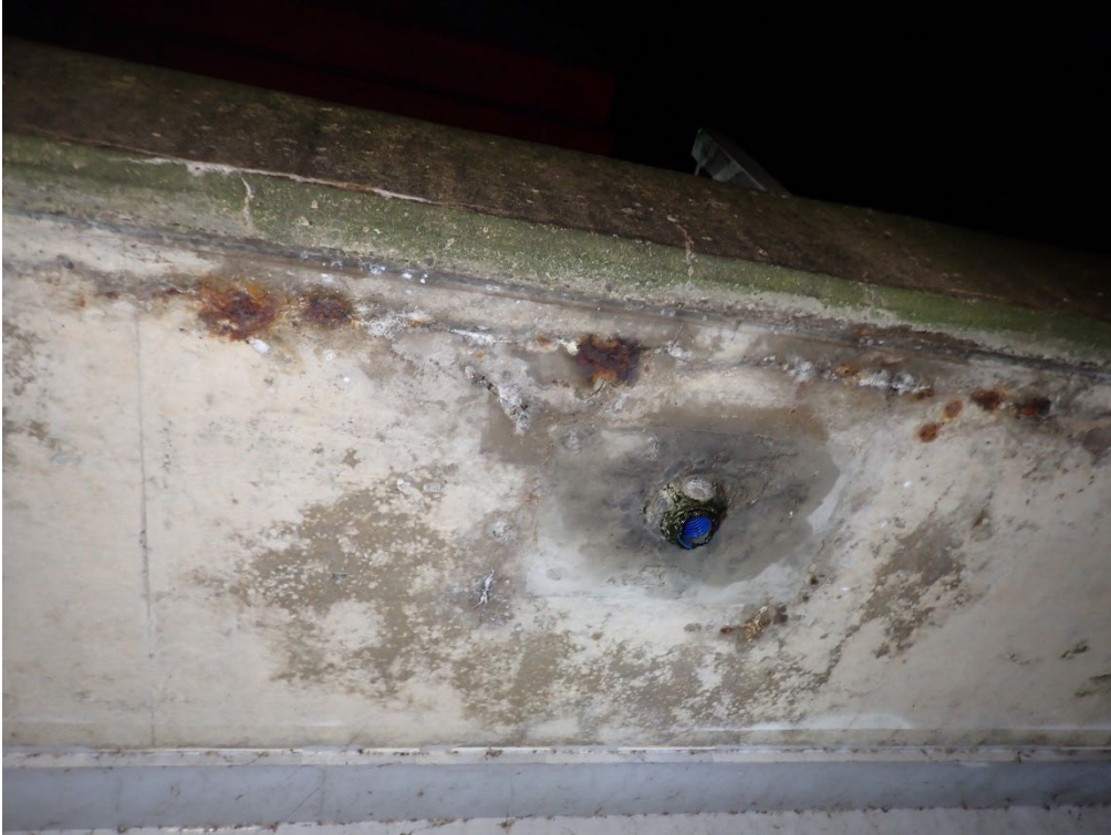
Plate 111. Rust staining to the North edge beam, inner East span
