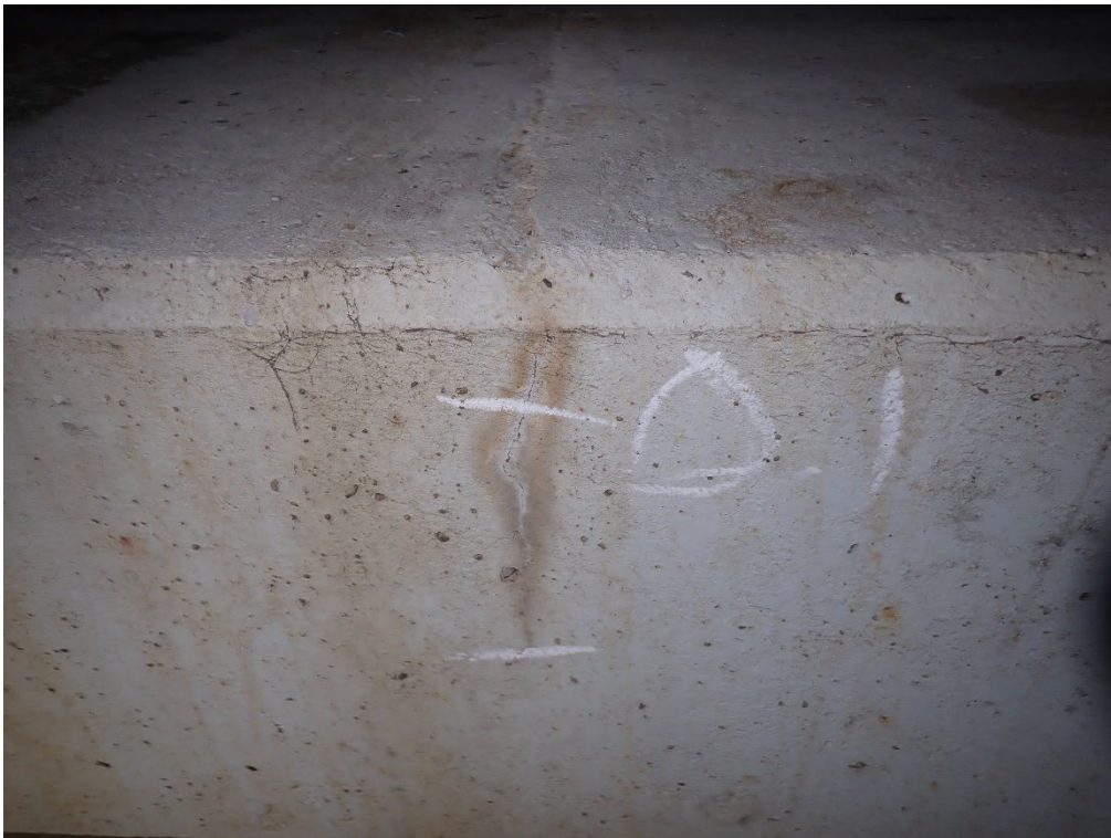
Plate 68. Cracking to the West Pier concrete cap
