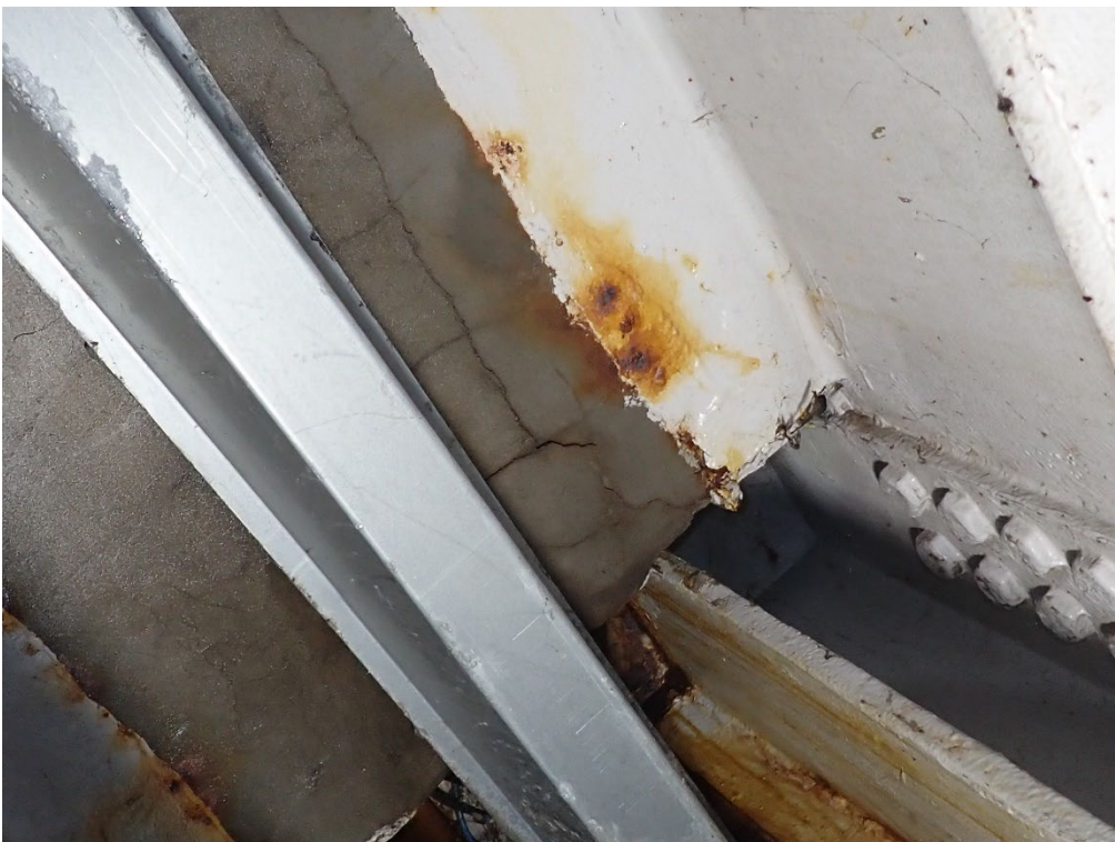
Plate 138. Cracking and delamination to the repair beneath the Centre Pier joint
