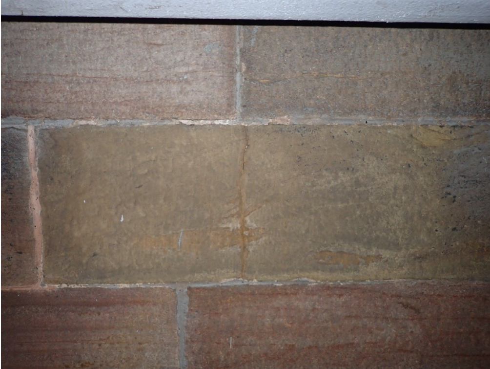
Plate 49. Fine cracking through stones in the East Abutment back wall
