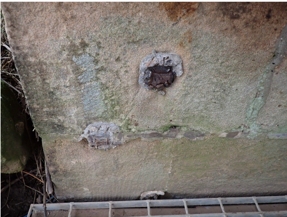
Plate 48. Corroded historic fixings in the East Abutment
