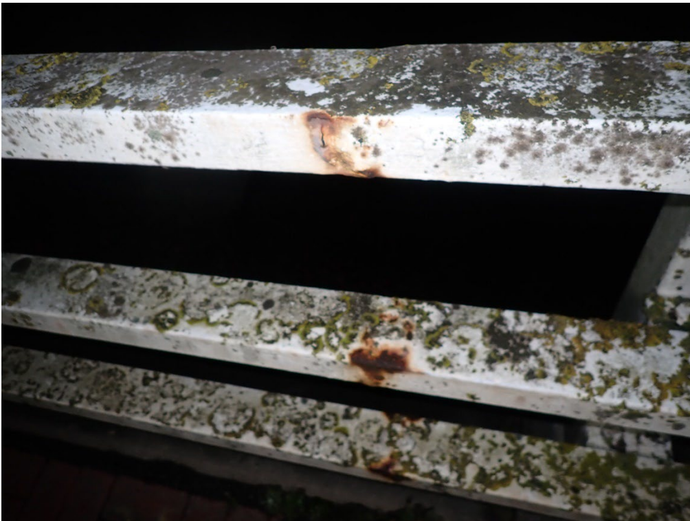
Plate 166. Typical corrosion to North Parapet rails where paintwork has failed
