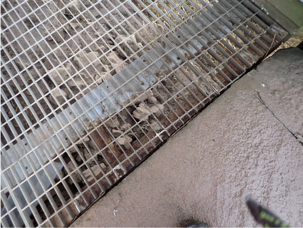
Plate 179. Corrosion to the topside of the Walkway supports
