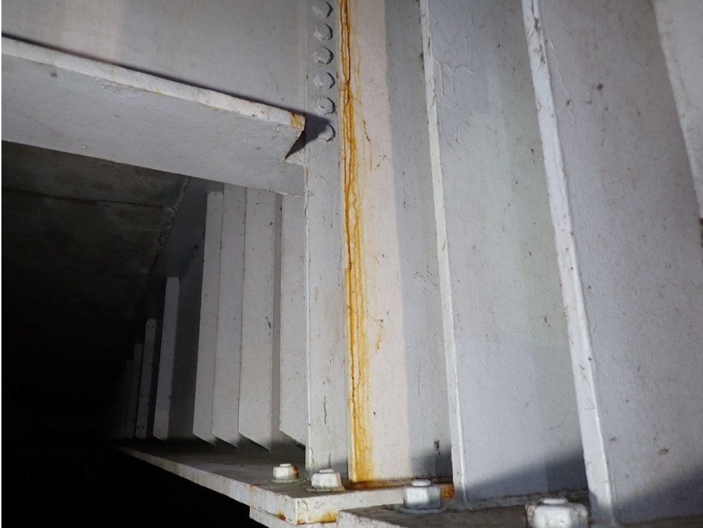
Plate 99. Corrosion Staining to steelwork above the West Pier
