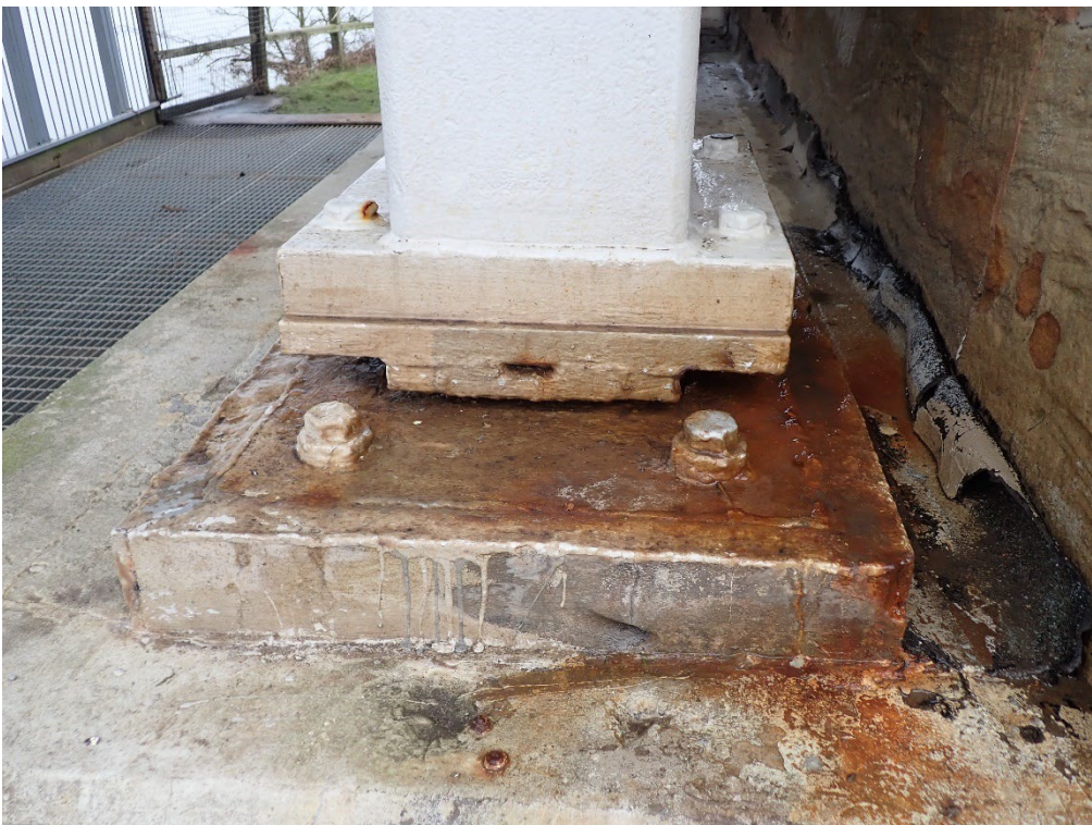
Plate 82. Rust staining to East Abutment bearing (South)
