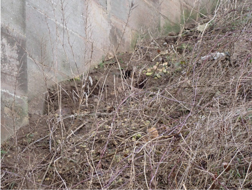
Plate 171. Animal burrows on the bank adjacent to the South-West Wing Wall
