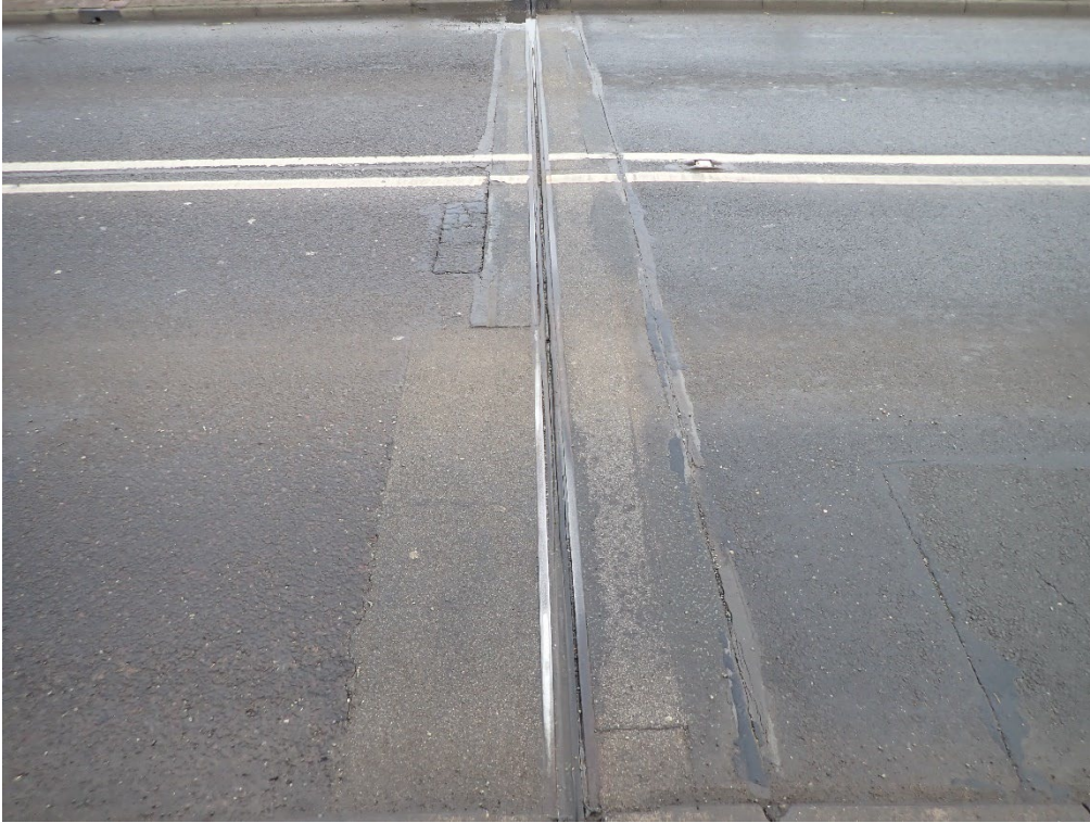
Plate 155. Deformed seal on the East joint
