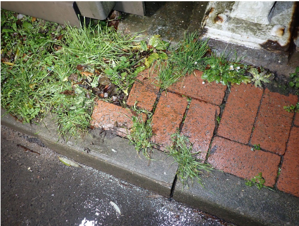
Plate 160. Misaligned bricks at the West End of the North Verge
