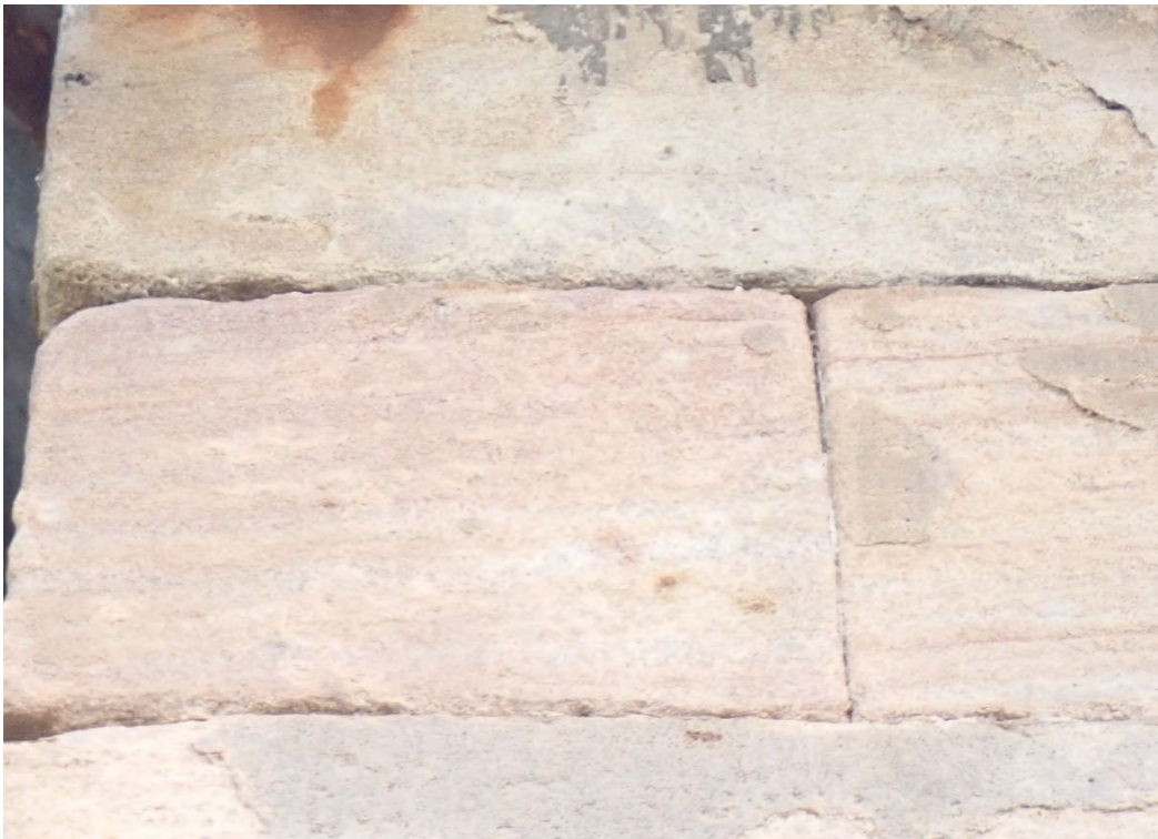
Plate 62. Mortar loss towards the top of the South-East wing wall
