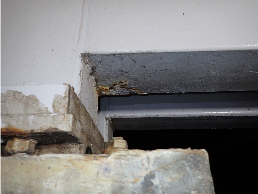
Plate 89. Paint blistering on the East Pier cross beam
