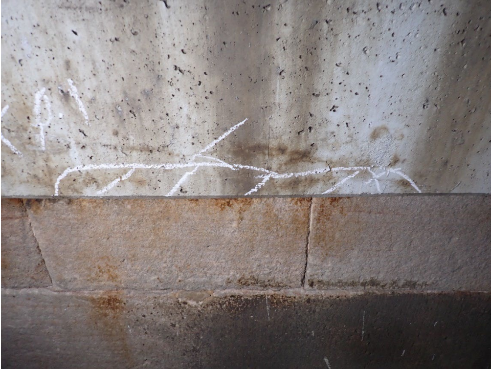
Plate 65. Reinforcement corrosion cracking with adjacent delamination 770 x 80mm, Centre Pier
