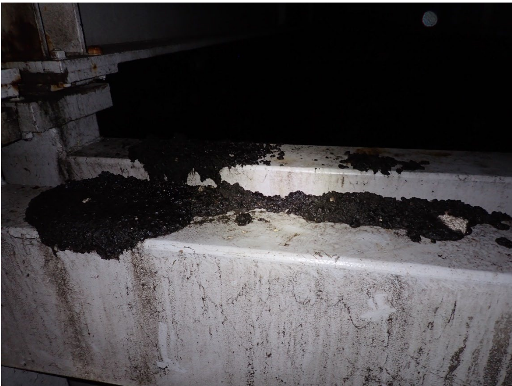
Plate 104. Bitumen on the transverse beam of the Centre Pier, from repairs at the Centre Joint
