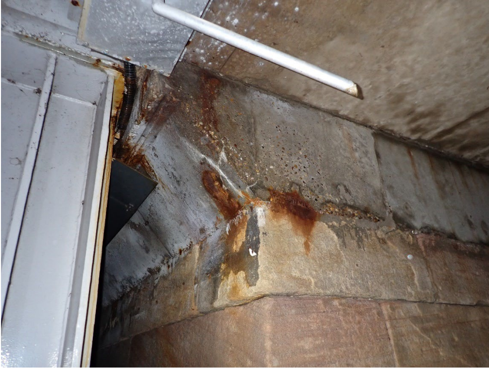
Plate 61. Rust Staining to Slab above South-East Wing Wall
