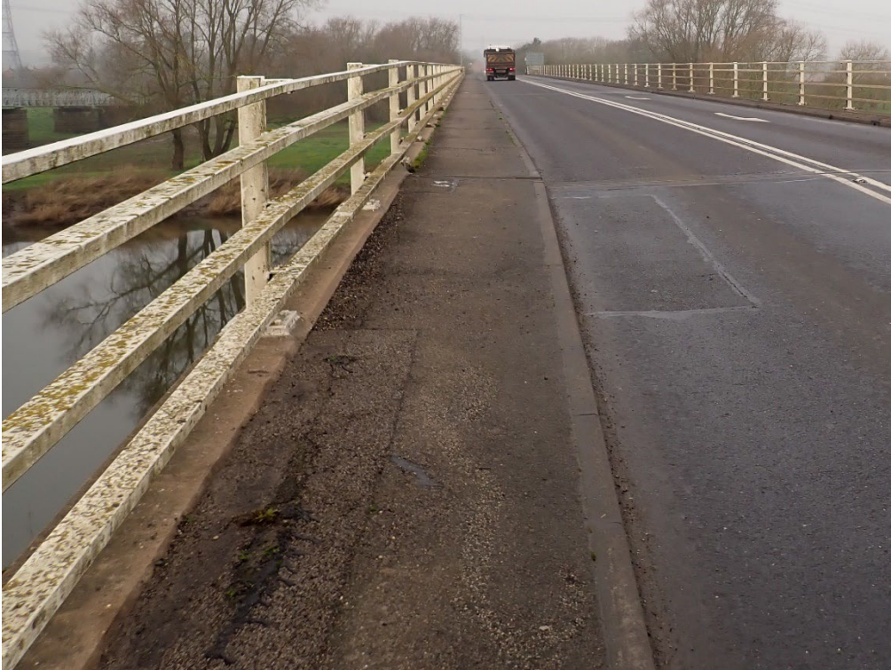
Plate 159. Cracking on the East Approach of the South footpath
