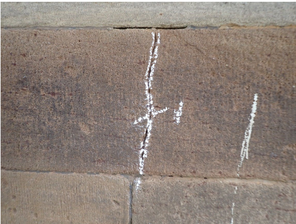
Plate 78. Cracking 1mm wide to the West Pier
