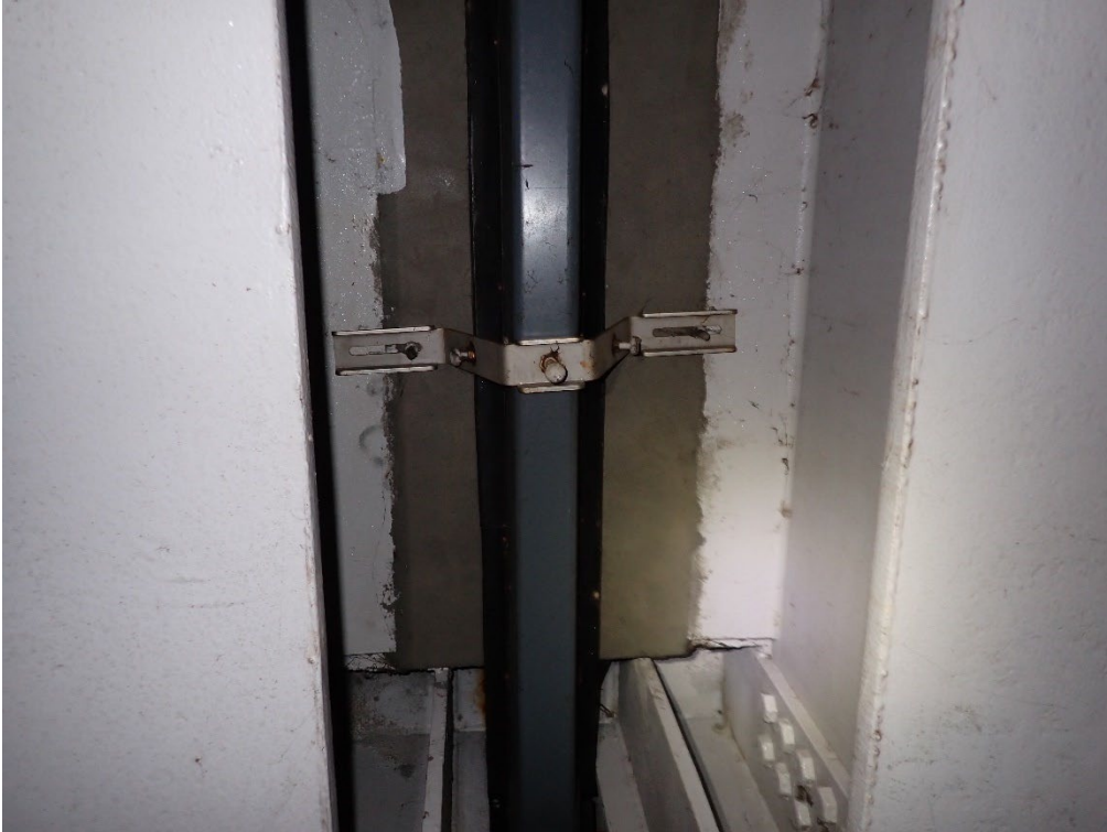
Plate 141. Water-stained repair on the south end of the East Pier joint
