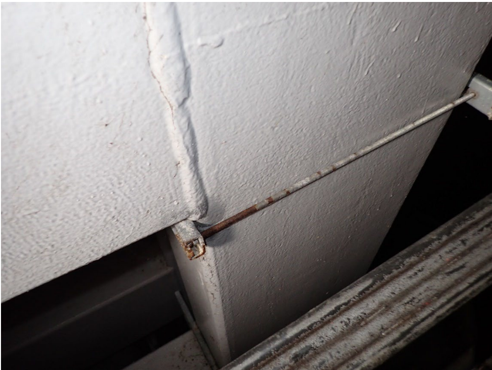
Plate 130. Minor corrosion to downpipe fixing on the Centre Pier
