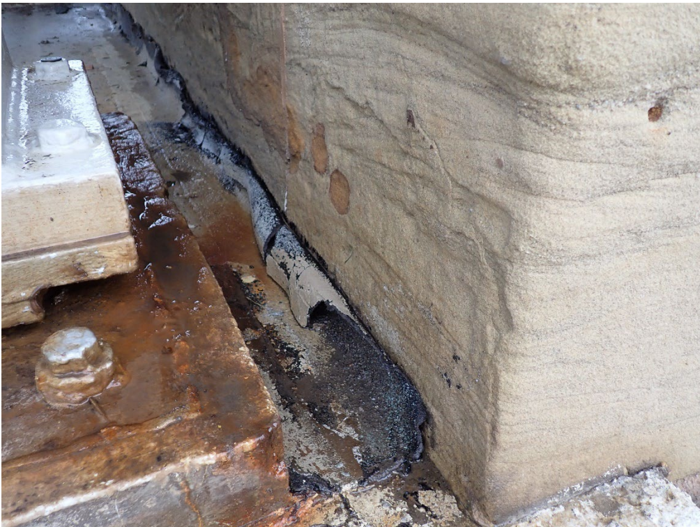
Plate 54. Damage to felt on the East Abutment
