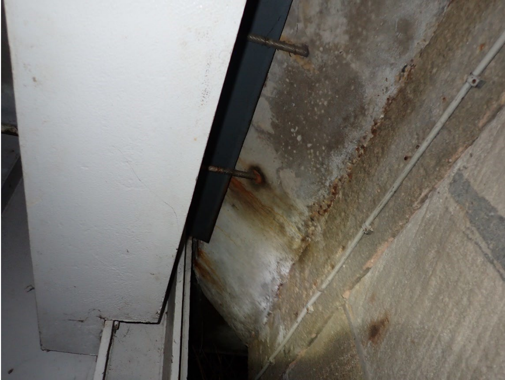
Plate 41. Rust staining emanating from the drainage deflector on the West Abutment, south end
