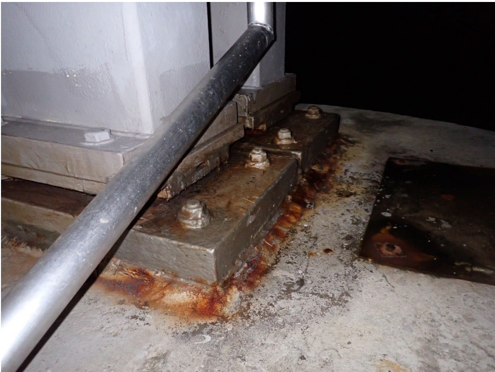
Plate 84. Rust staining to lower bearing on the West Pier
