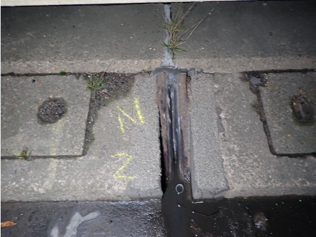
Plate 125. De-bonding of sealant above the West Pier, North edge beam
