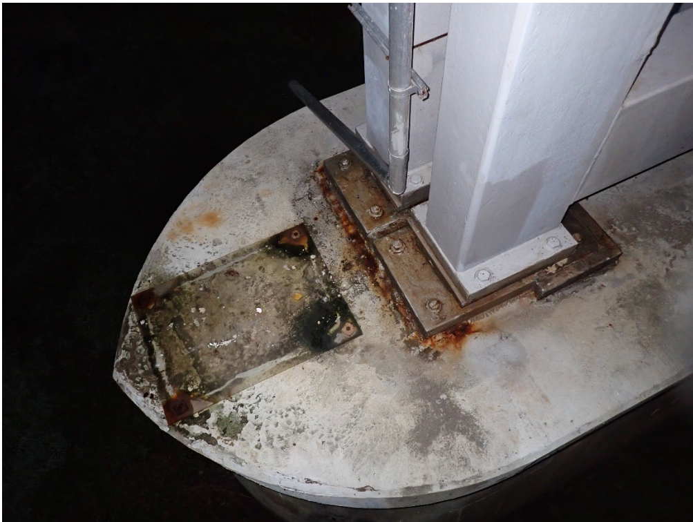
Plate 74. Water-stained downstream end of the West Pier
