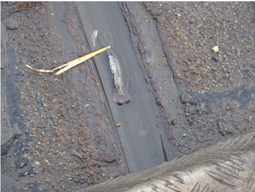
Plate 142. Active water ponding in the West Joint
