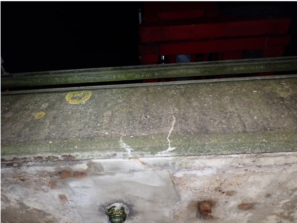
Plate 120. Typical cracking to North edge beam on inner East Span
