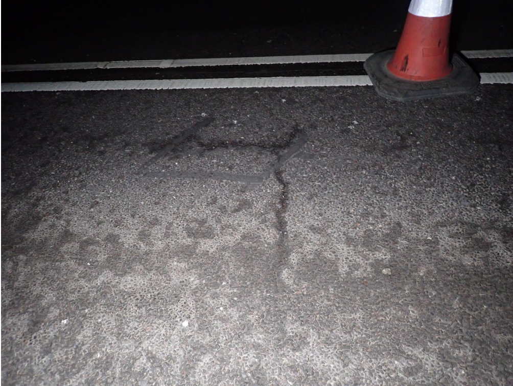
Plate 135. Open and sealed cracks in surfacing on the East Span
