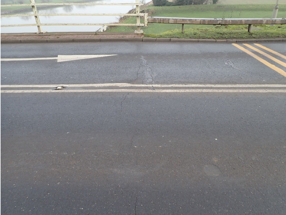
Plate 133. Settlement and transverse cracking on the West Approach
