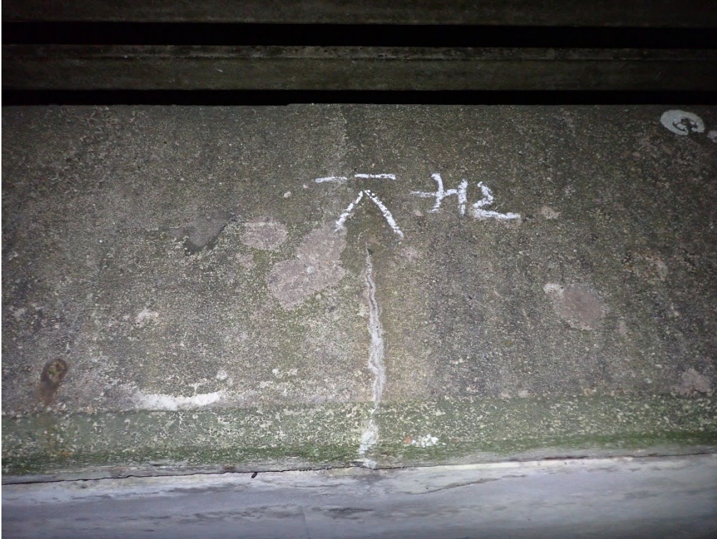
Plate 119. Crack with leachate to the West Span edge beam
