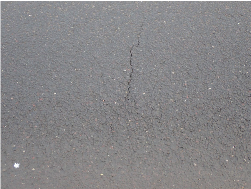
Plate 134. Open crack in surfacing on the West Span
