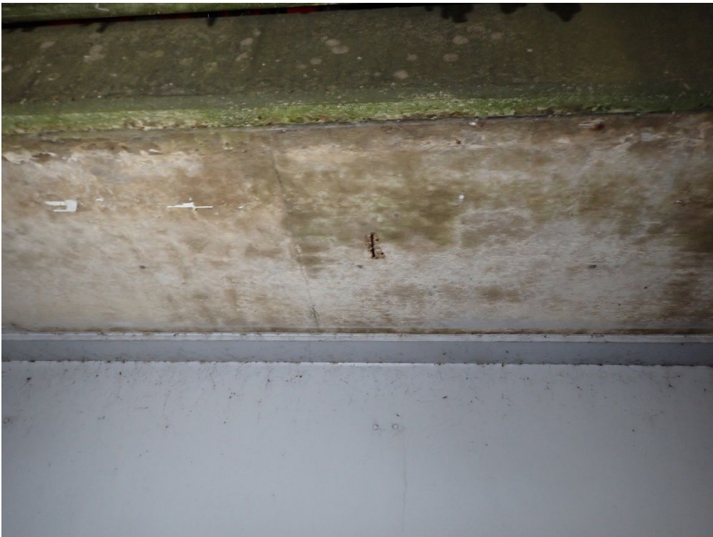
Plate 116. Spalled concrete exposing reinforcement in North Cantilever soffit, East Span
