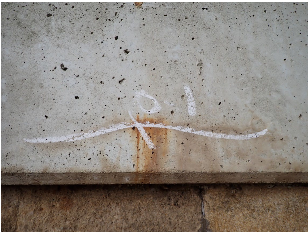
Plate 38. Reinforcement corrosion cracking to West Abutment concrete cap
