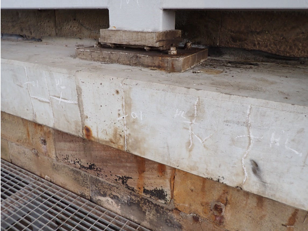
Plate 39. Reinforcement corrosion cracking to East Abutment concrete cap.
