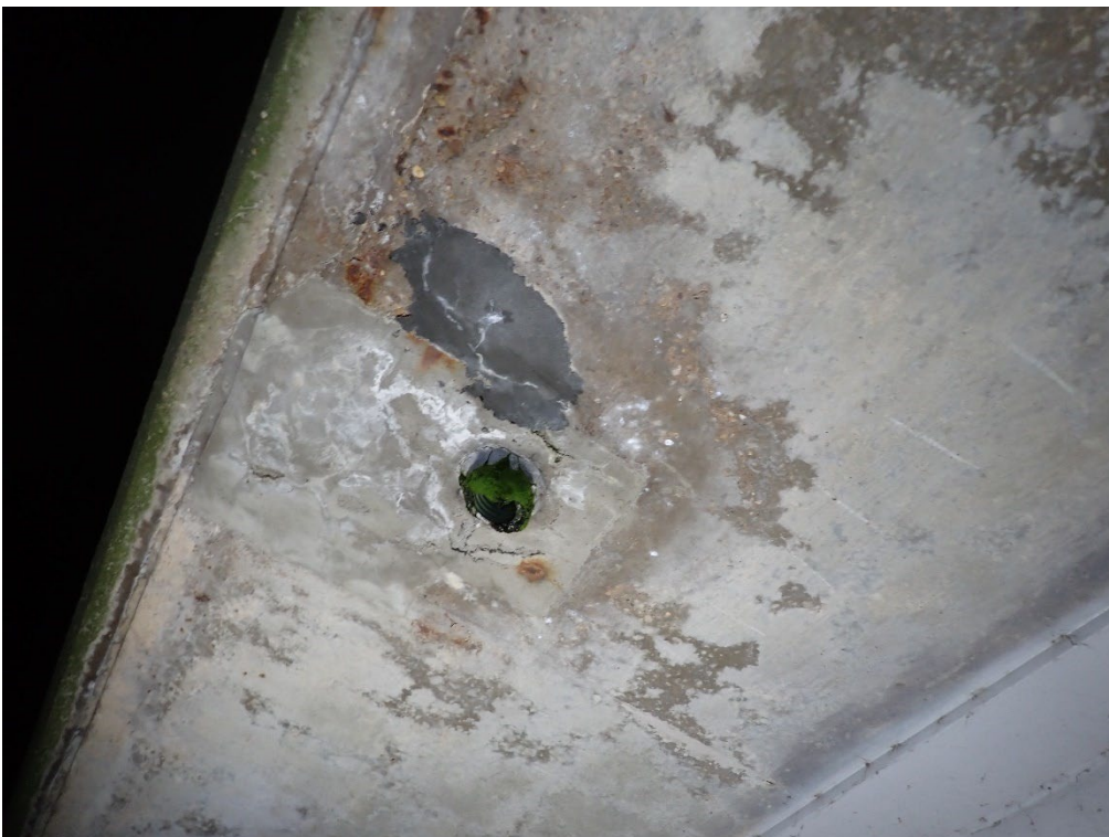
Plate 112. Rusty tie wire and repair to the North edge beam, inner West Span
