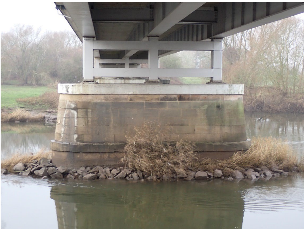
Plate 76. Calcite Deposits to the Upstream End of the East Pier
