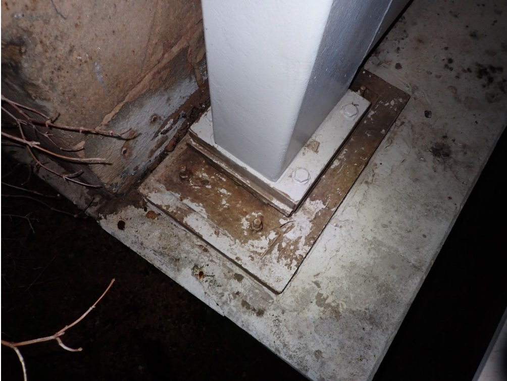
Plate 85. Protective paint loss on the West Abutment lower bearing
