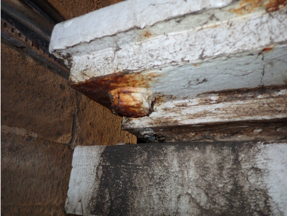
Plate 83. Rust staining to upper connection of upper Bearing, West Abutment
