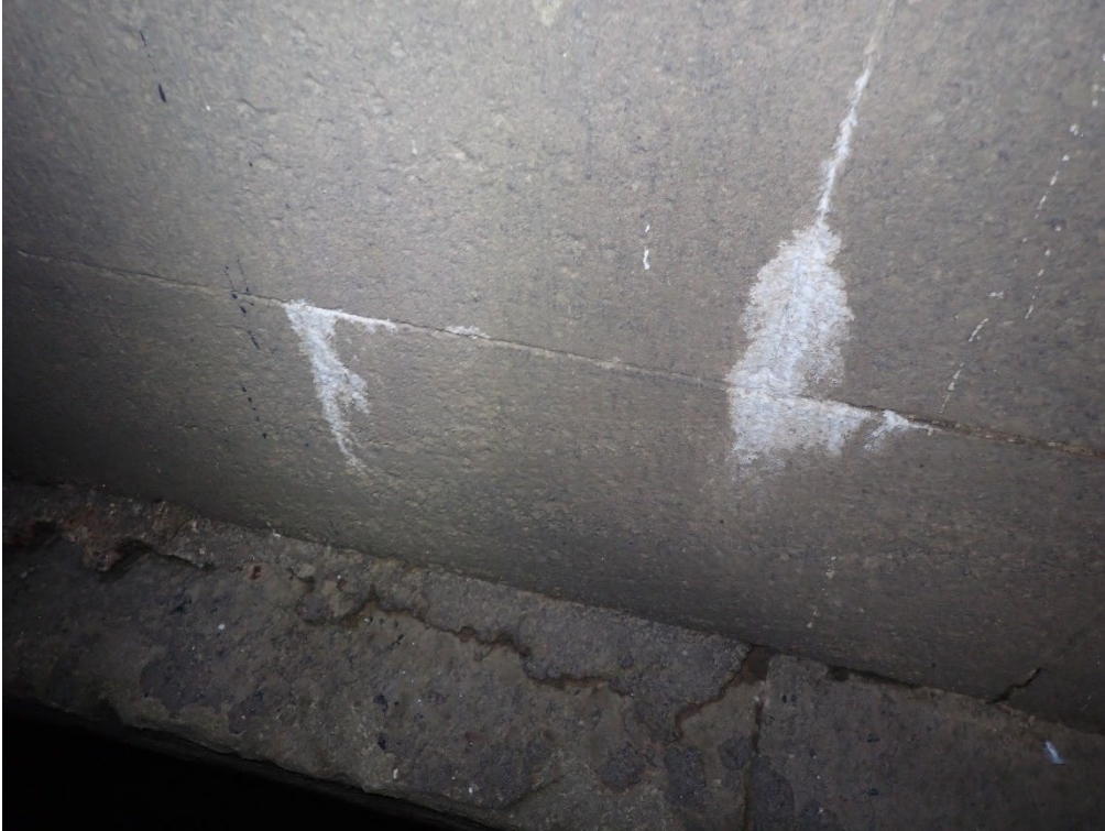
Plate 77. Leachate through mortar joints within the Centre Pier
