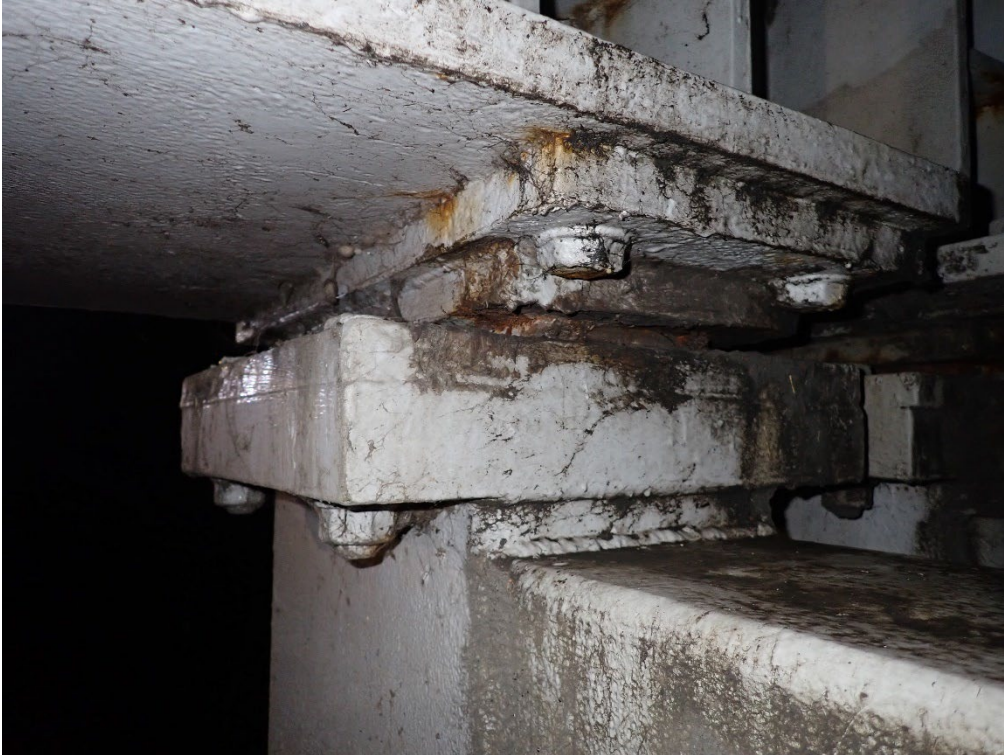
Plate 87. Rust staining to the upper bearing on the West Pier
