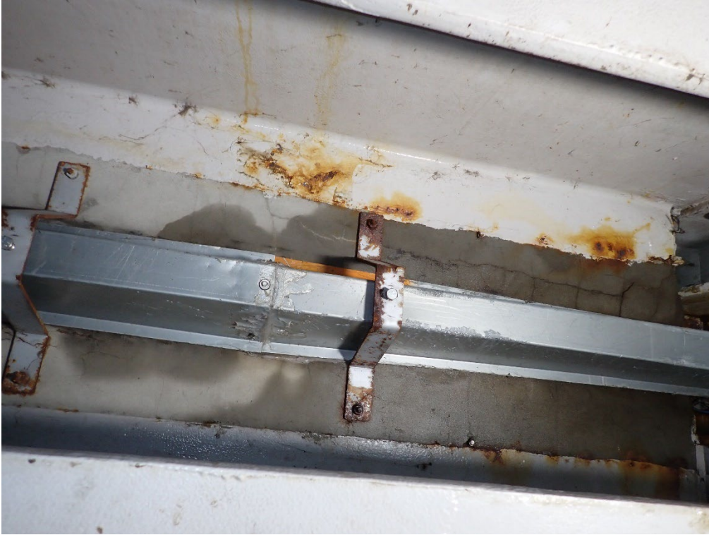
Plate 101. Corrosion to transverse beam at the Centre Pier
