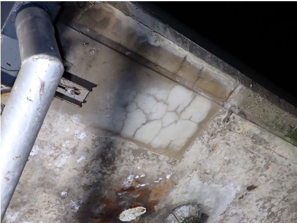
Plate 114. Cracks to concrete repair at East Joint
