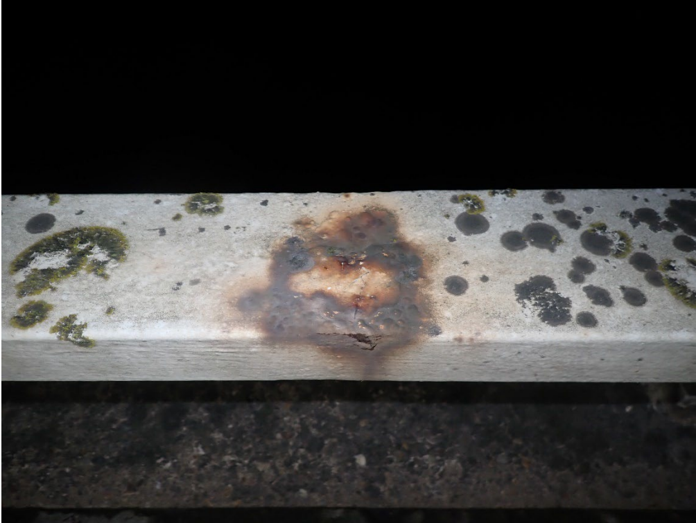
Plate 167. Area of paint loss to the North Parapet where corrosion has occurred
