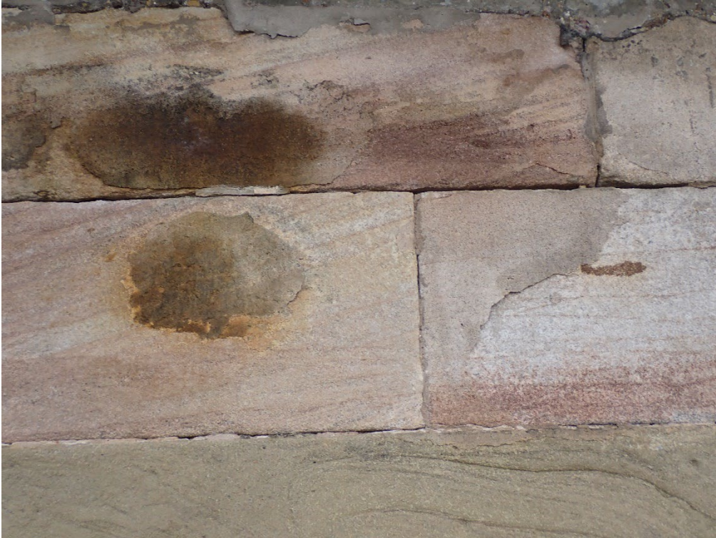
Plate 53. Mortar loss between the East Abutment brickwork
