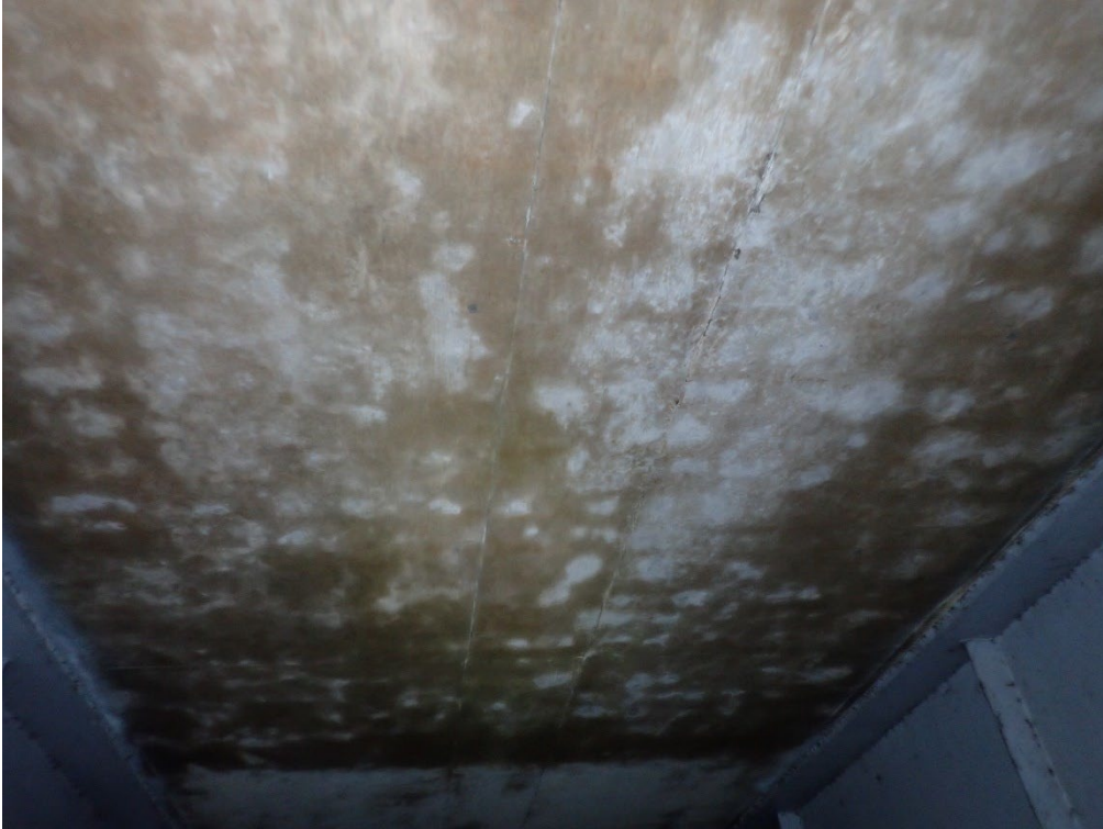
Plate 131. Water staining to the East Span adjacent the East Pier
