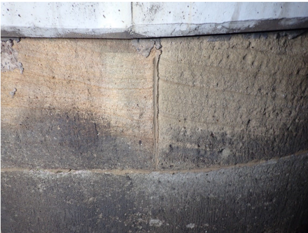
Plate 80. Mortar loss to the East Pier
