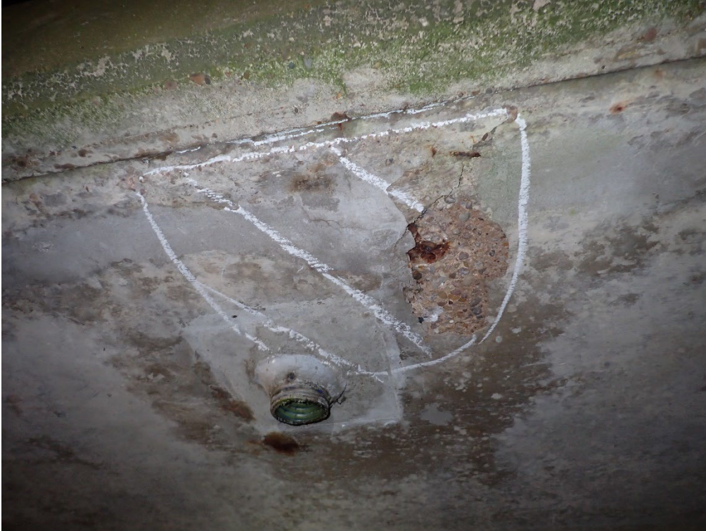
Plate 105. Delamination to the South edge beam on the West Span, 450 x 430mm
