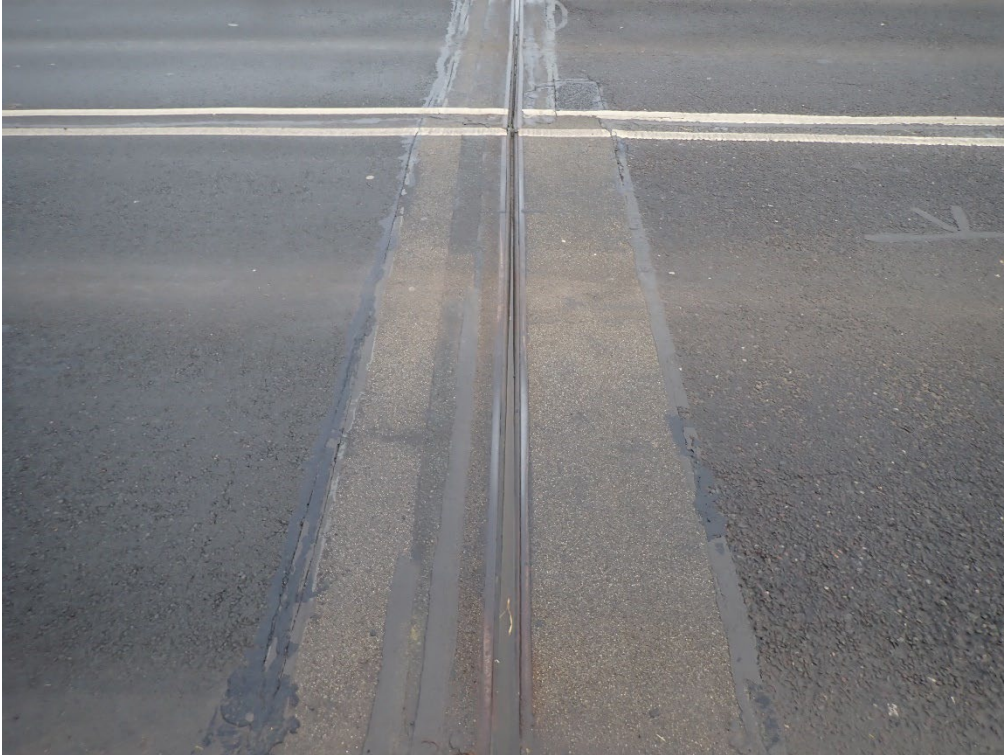
Plate 145. Failed repair to cracking adjacent to the West Abutment Joint
