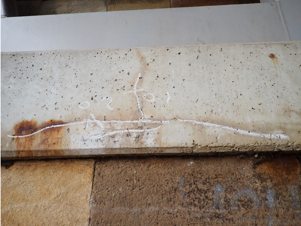
Plate 37. Reinforcement corrosion cracking to West Abutment concrete cap
