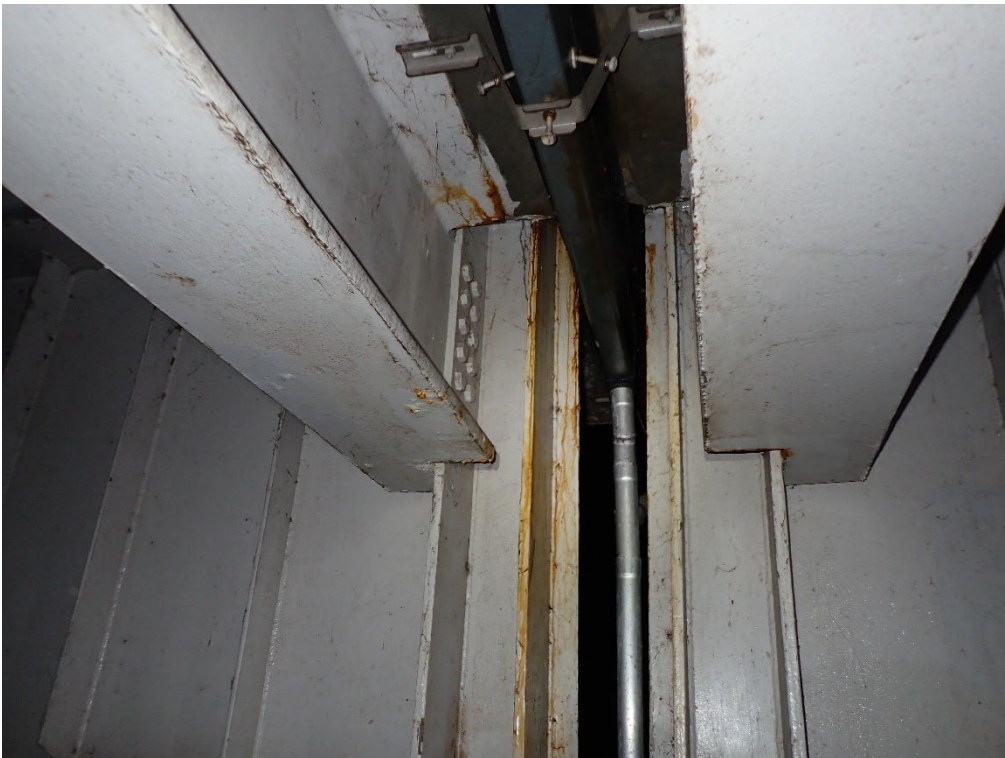
Plate 102. Corrosion staining to the transverse beam over the West Pier
