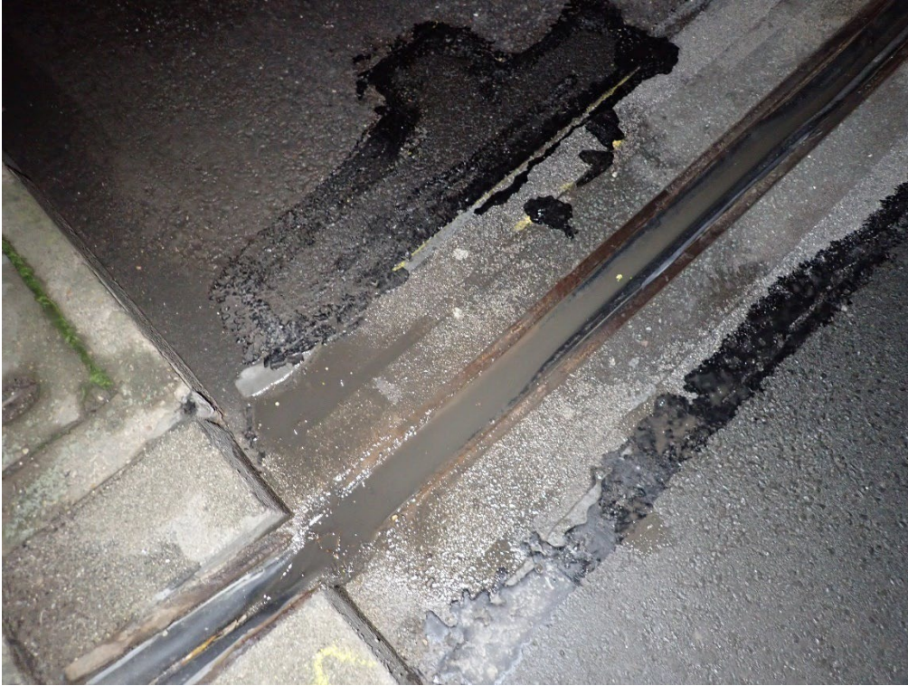
Plate 143. Active water ponding in the Centre Pier joint
