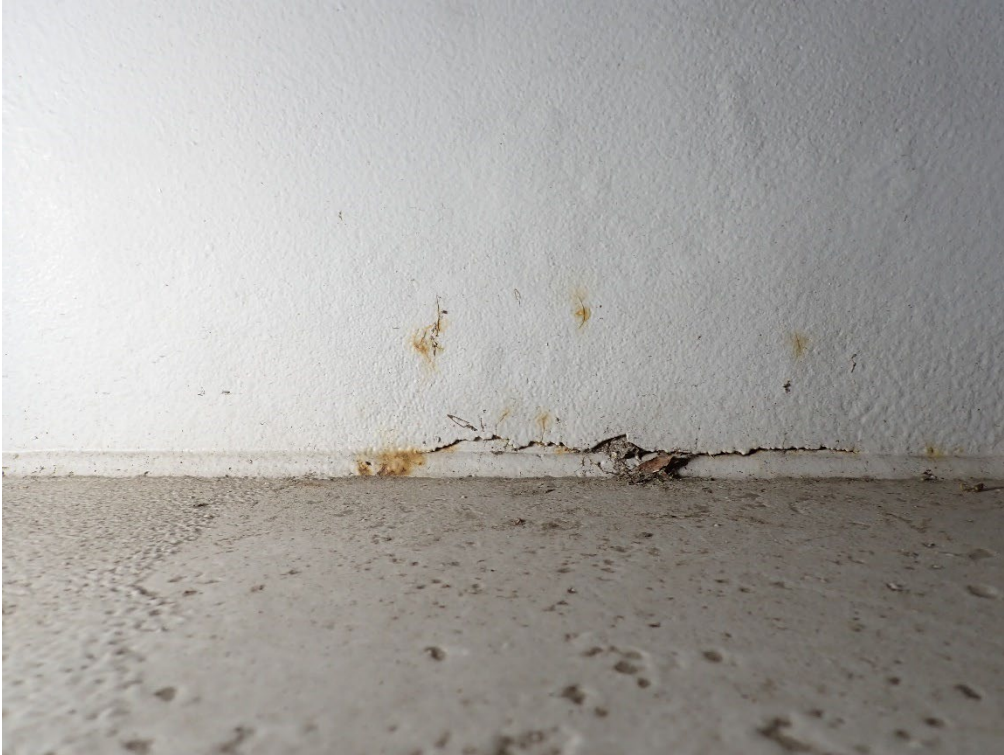
Plate 97. Cracked paint to the North beam on the inner West Span
