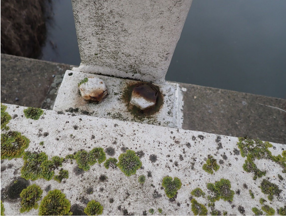
Plate 165. Typical Corrosion to Fixings Where Paint Has Failed
