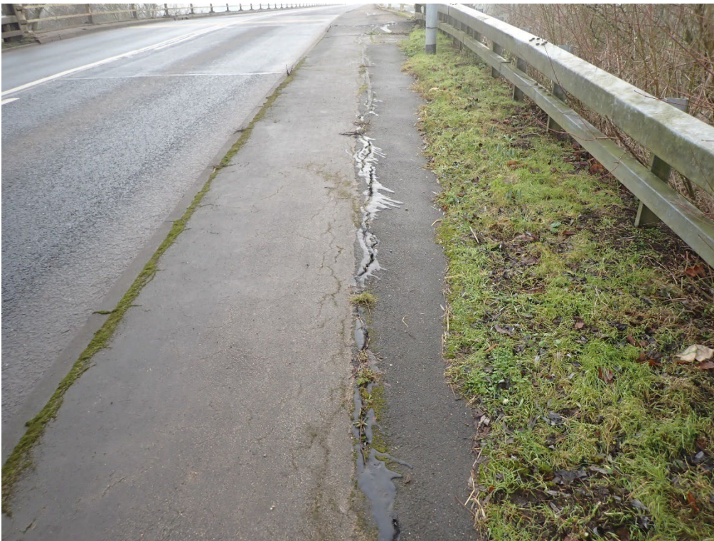
Plate 158. Cracking to a repair on the West end of the South verge on the approach
