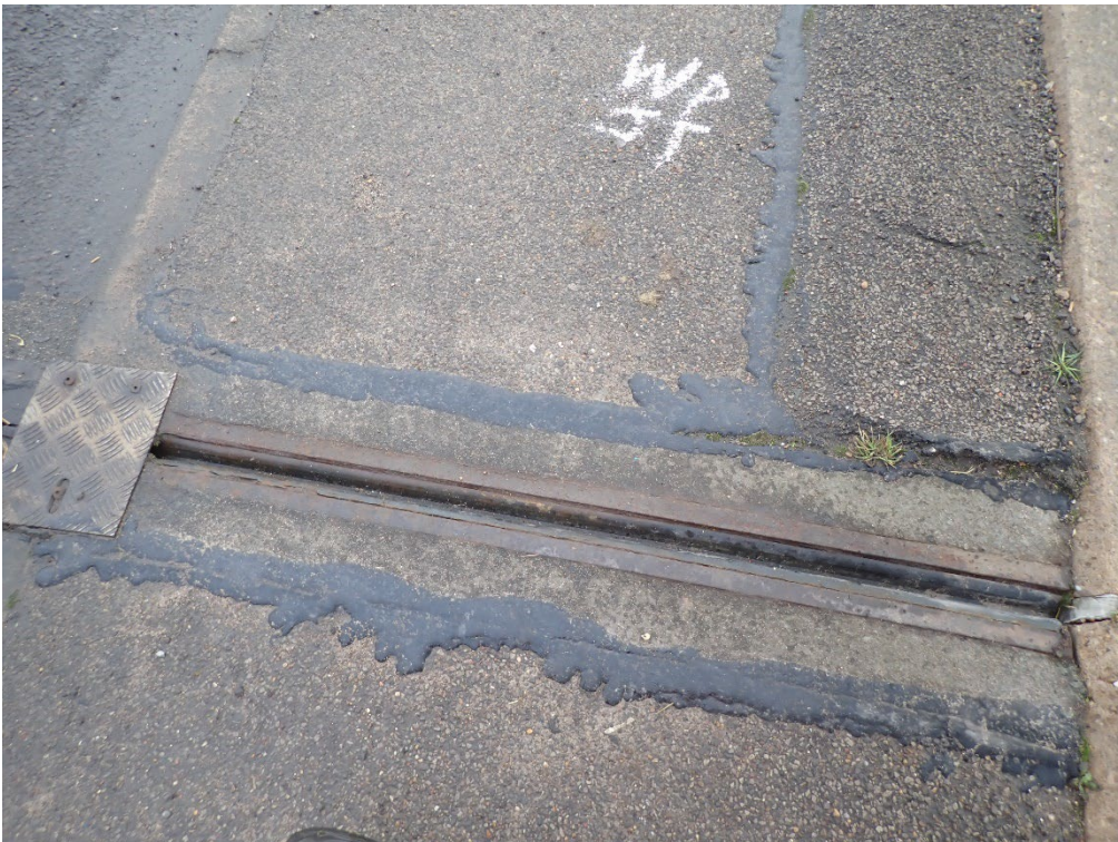
Plate 150. Corrosion to the West Pier Joint nosing rails
