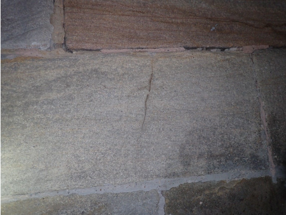
Plate 51. Fine cracking through stones in the West Abutment back wall
