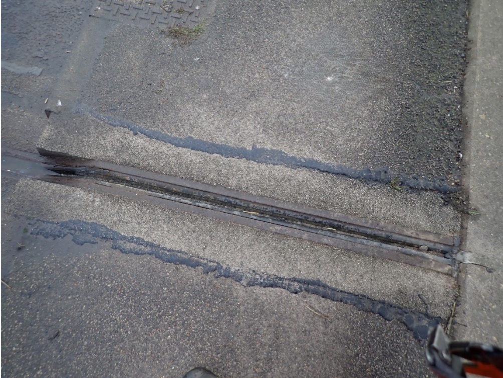
Plate 151. Corrosion to Nosing Rails of the Centre Pier Joint
