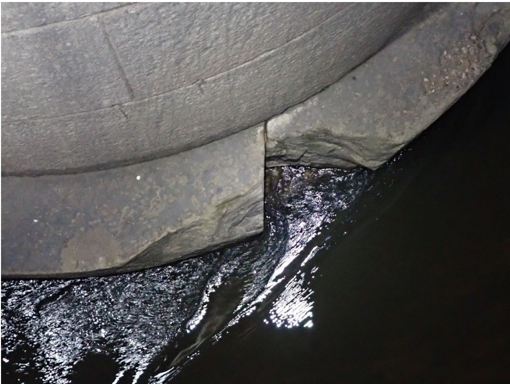
Plate 72. Impact Damage to Upstream End of the East Pier
