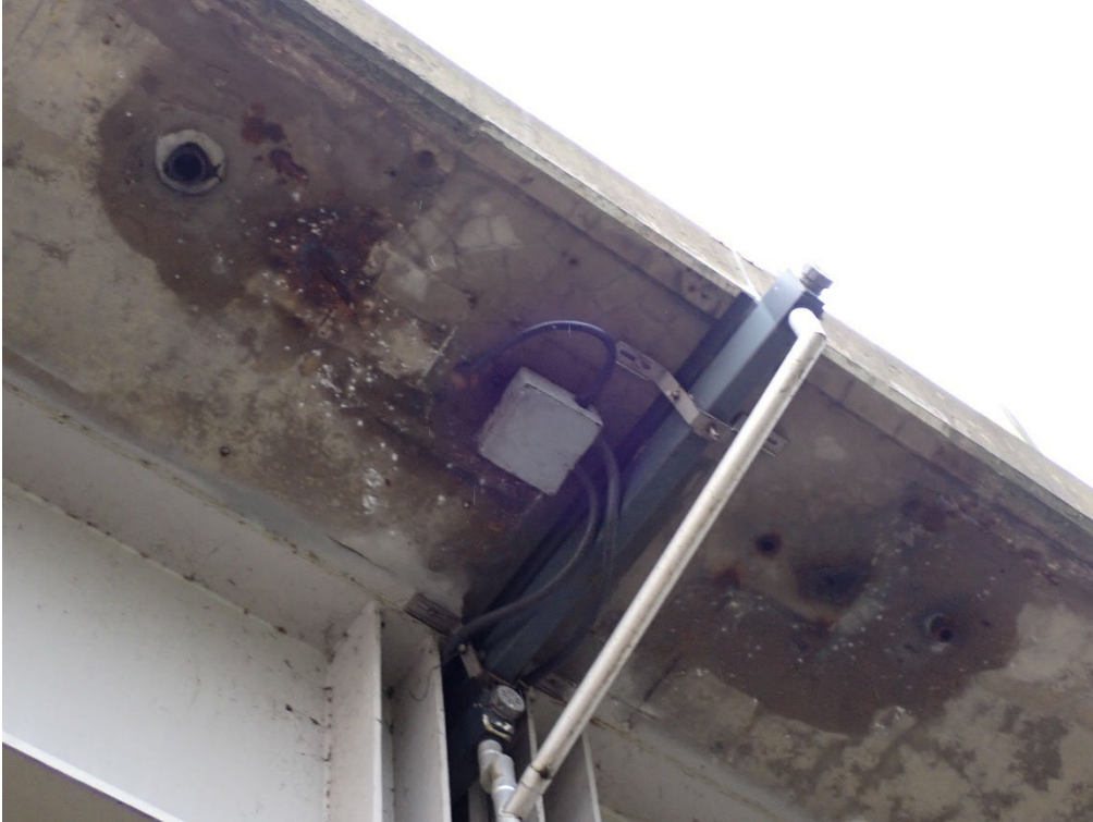
Plate 115. Water seepage to the deck soffit on the North end at the West Joint
