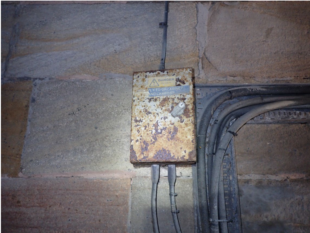
Plate 57. Open and corroded cathodic protection cabinet on the West Abutment back all
