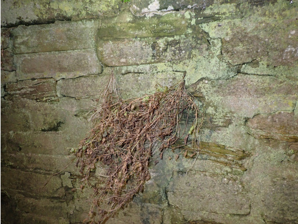
Plate 175. Vegetation growth from the mortar joints of the East Retaining Wall
