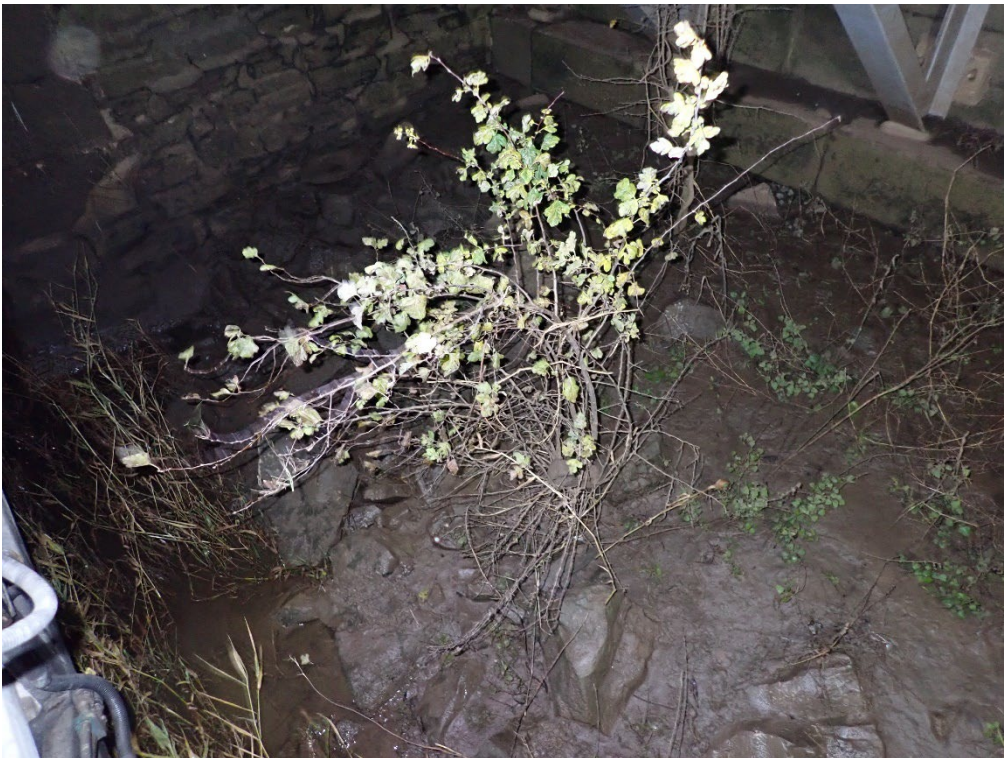
Plate 176. Tree growth between the two Retaining Walls beneath the East Abutment Walkway
