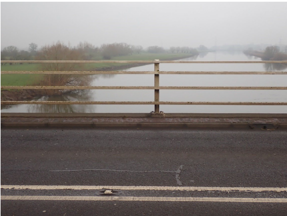
Plate 136. Sealed cracks in surfacing on the Inner East Span
