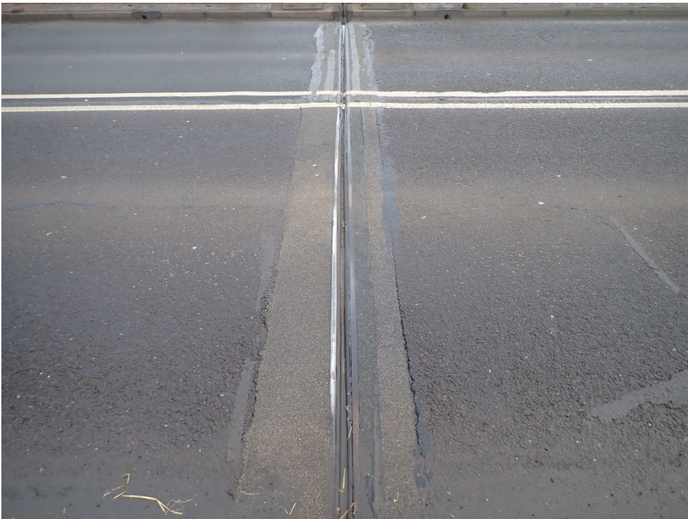
Plate 146. Debonding between the nosing surfacing and carriageway, West Pier joint
