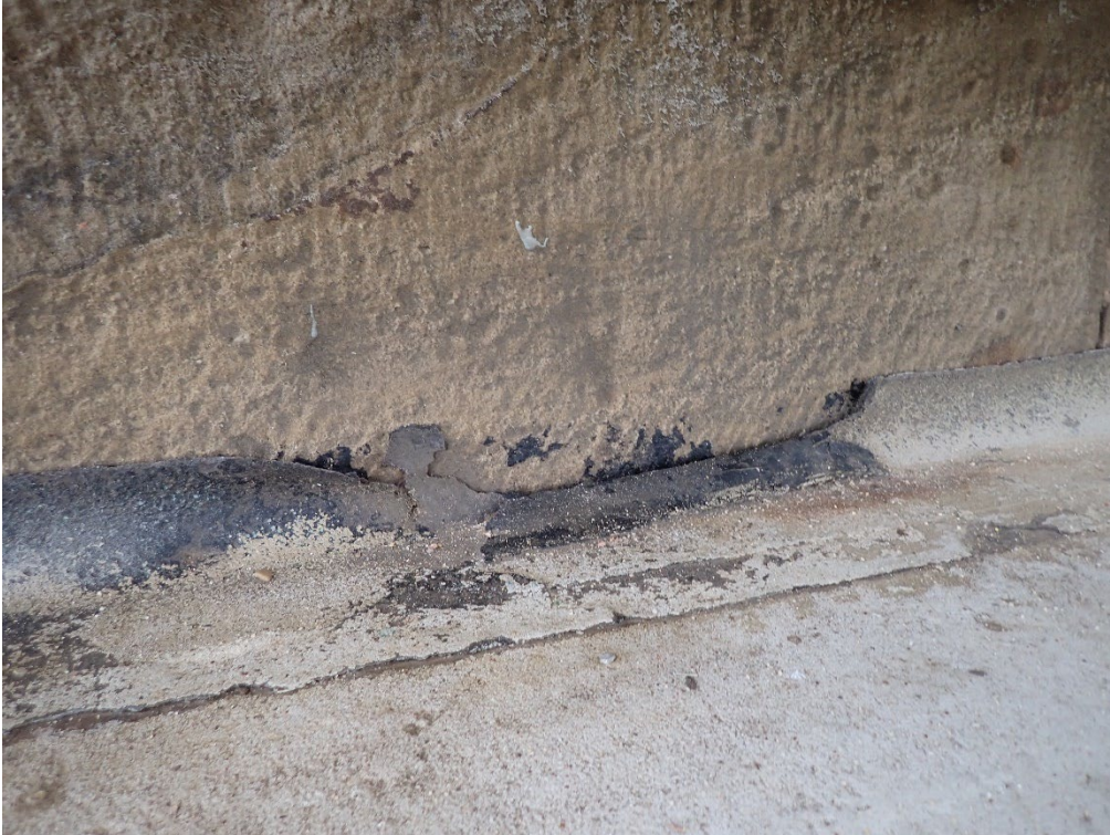
Plate 55. Damage to felt on the East Abutment
