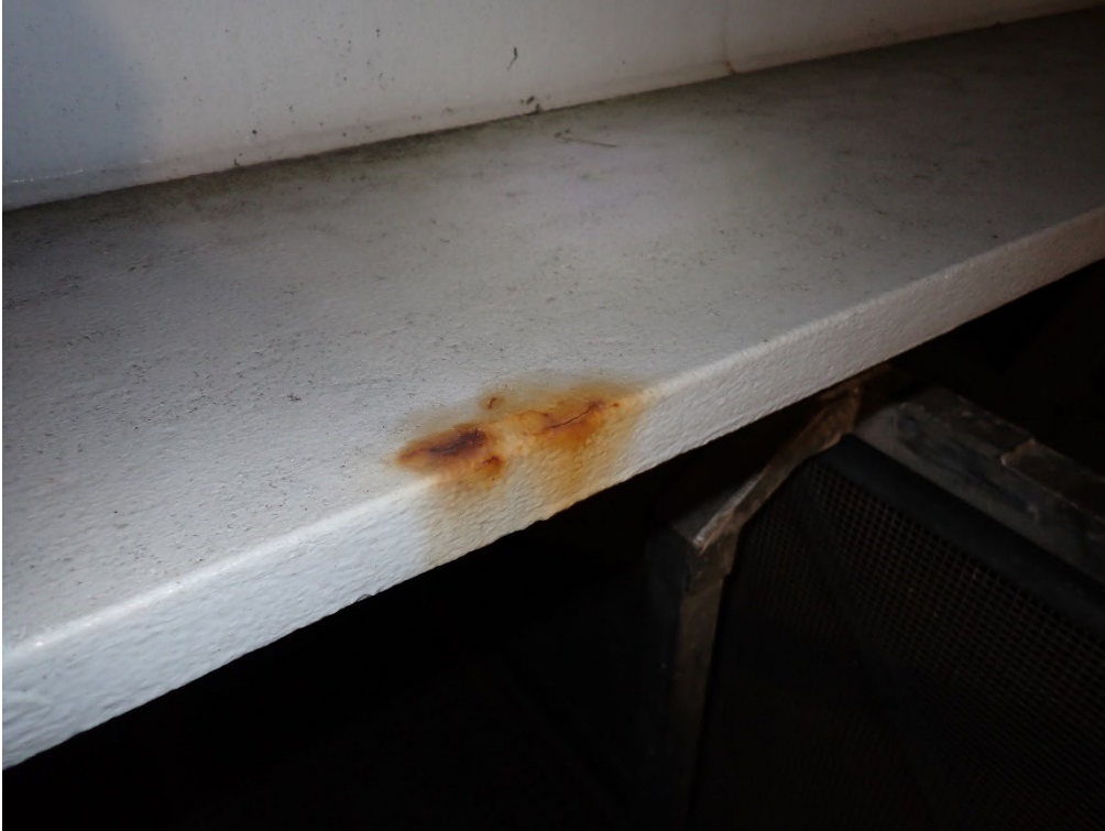
Plate 95. Flaking paint and minor underlying corrosion to North Beam, West Span
