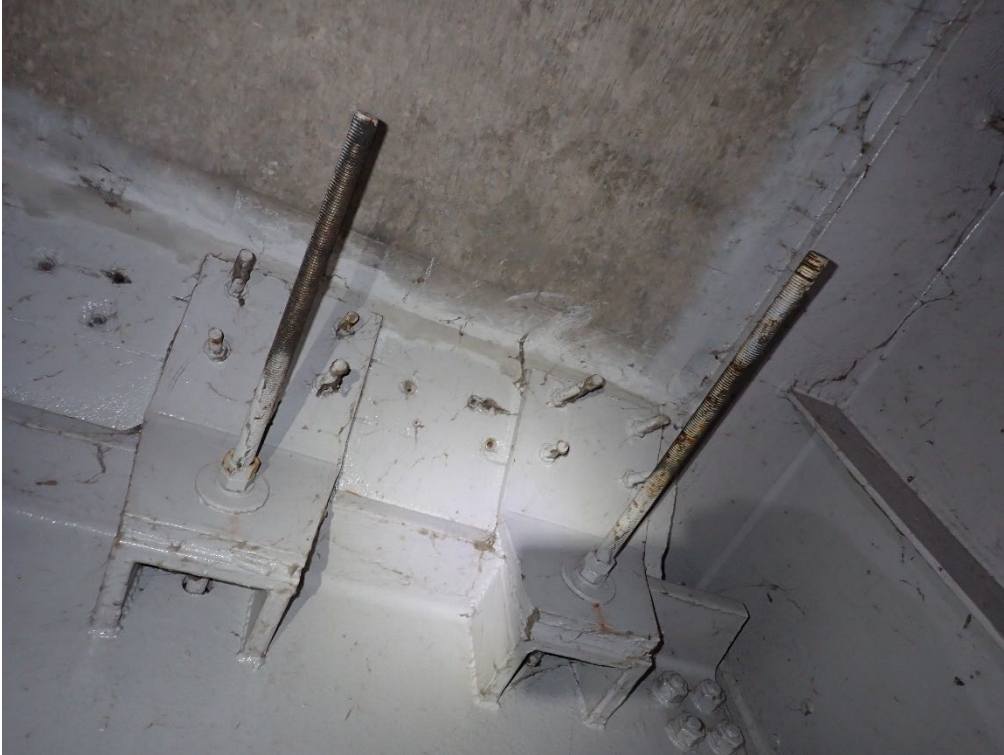
Plate 43. Exposed anchorage bars at the West Abutment, partially painted
