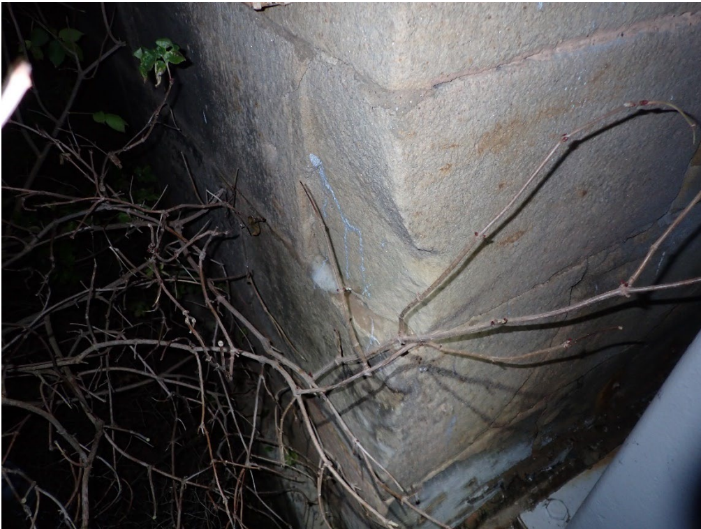
Plate 46. Shallow spall to the West Abutment, South end
