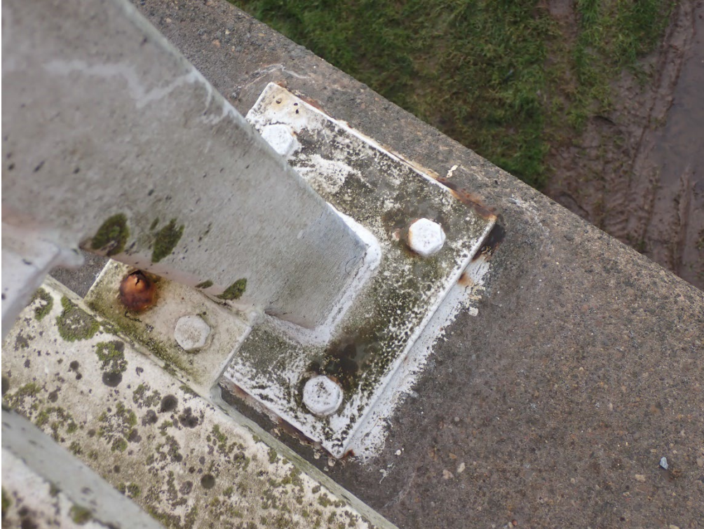
Plate 169. Typical cracking to Parapet base plate mortar
