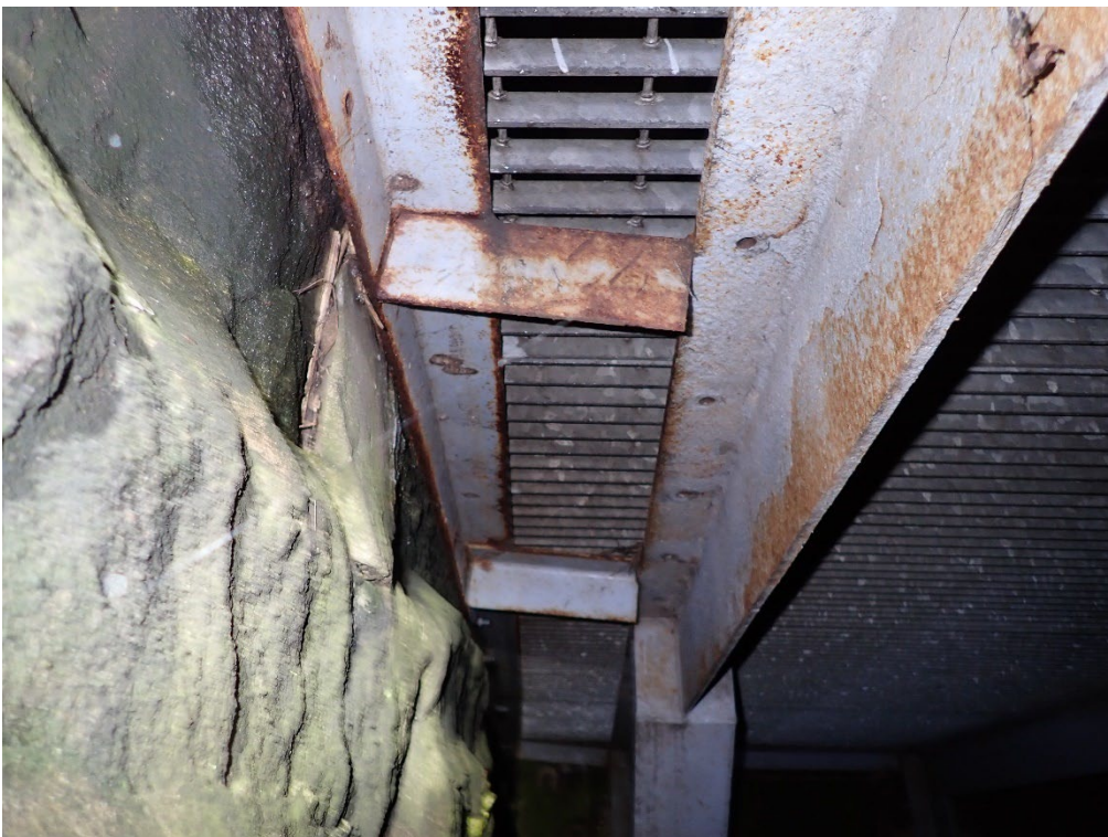
Plate 178. Minor corrosion to the underside of the Walkway
