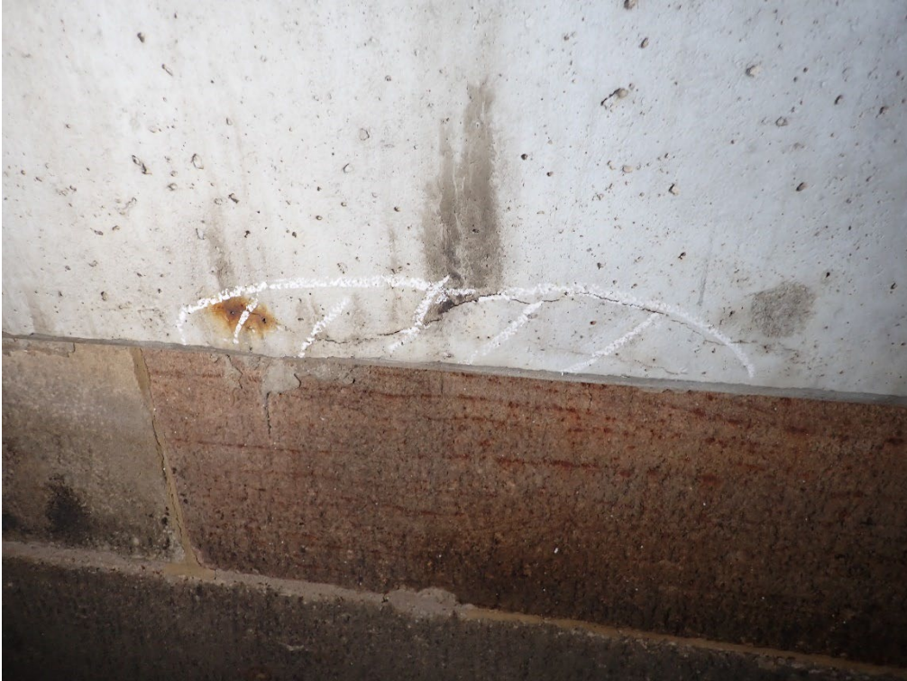
Plate 67. Delamination to the East face of the Centre Pier, 490 x 80mm with corrosion cracking
