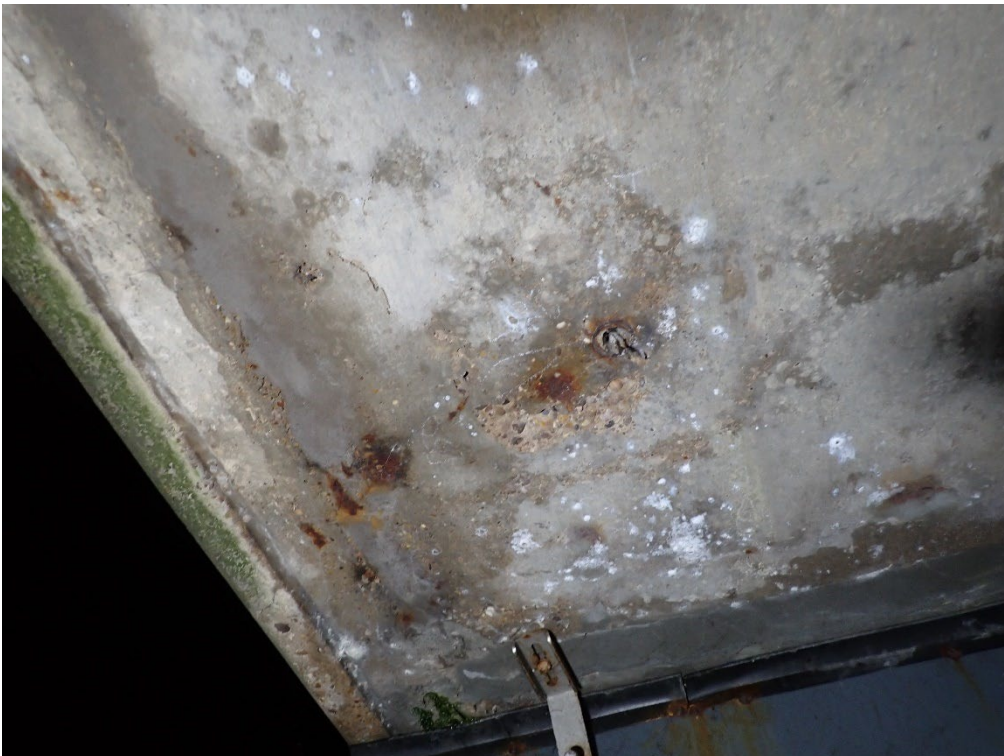
Plate 108. Minor delamination to the South edge beam adjacent the West Joint
