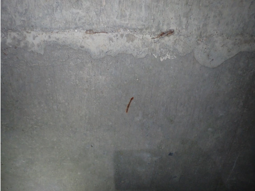
Plate 127. Minor corroded ferrous debris found in Deck Soffit, West Span
