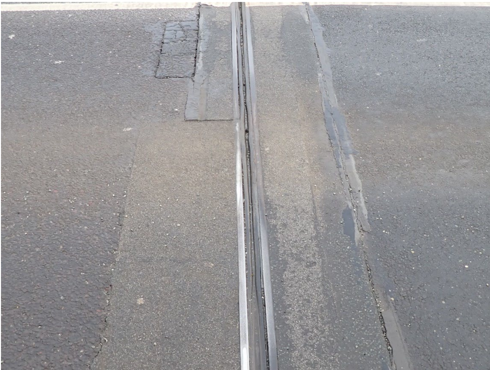
Plate 154. Deformed Seal in the East Abutment Joint
